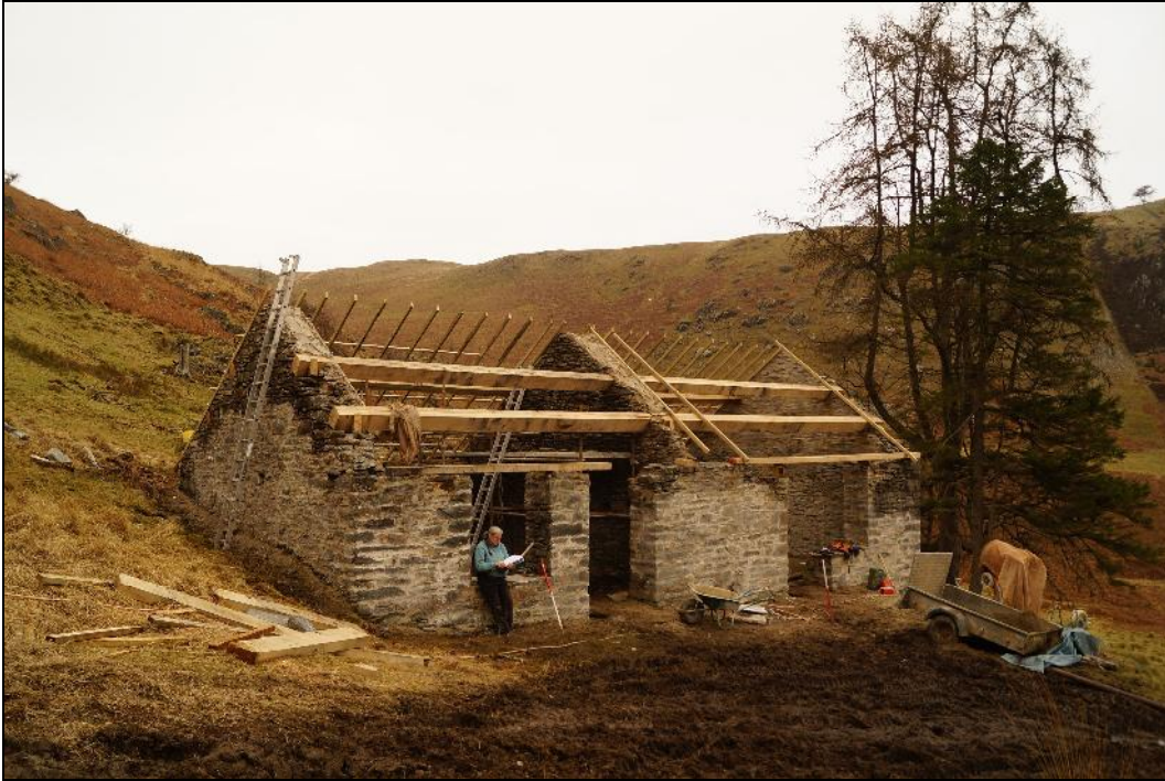
Plate 7: CEM2017_107. A view of the southern side of the former mine smithy building. Room A (the forge) is to the right and Room B to the left. Looking north-northeast.
