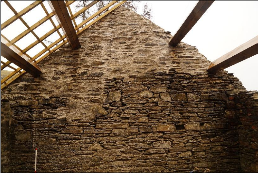
Plate 27: CEM2017_127. A view of the eastern gable wall of Room B. Looking east-northeast.
