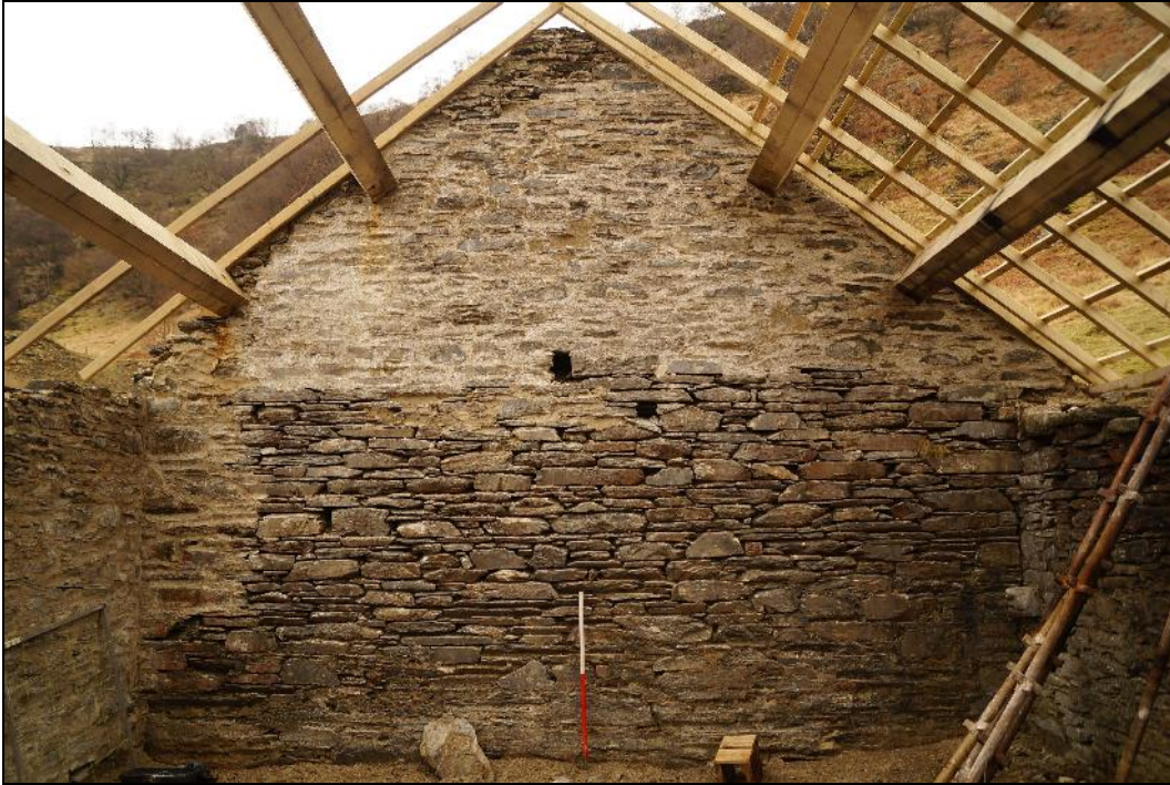
Plate 19: CEM2017_119. A view of the inside of the western gable wall of Room A. Looking west-southwest.
