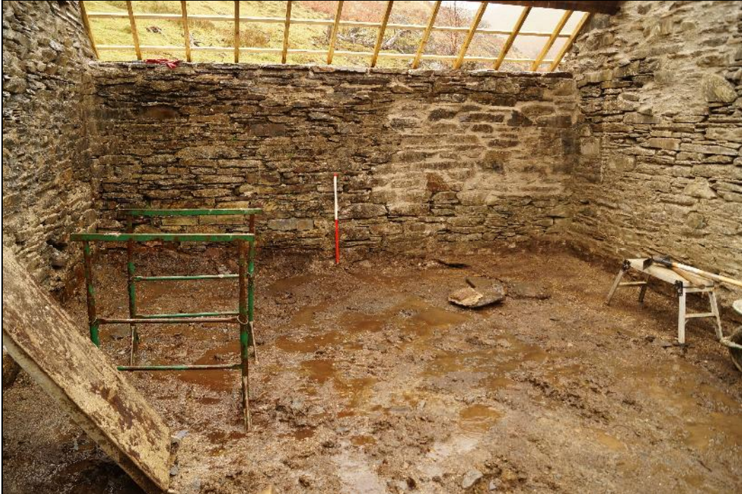
Plate 34: CEM2017_134. A view of the floor of Room B, after the removal of the mixed layer (007). The surface was quickly covered with waterlogged mud, with ground water flowing from the north wall towards the south wall. This level was maintained and terram and gravel was to be laid across the interior. Looking north.
