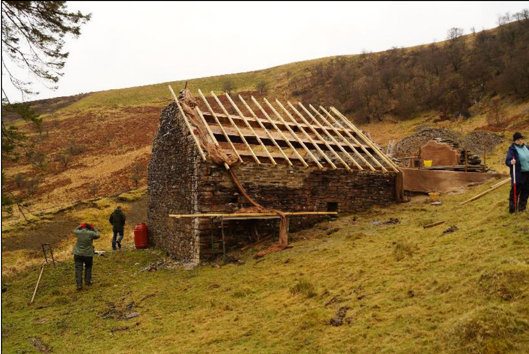
Plate 5: CEM2017_105. A view of the former mine smithy building. The spoil tips of the main shaft can be seen in the background to the right. Looking south-southwest.
