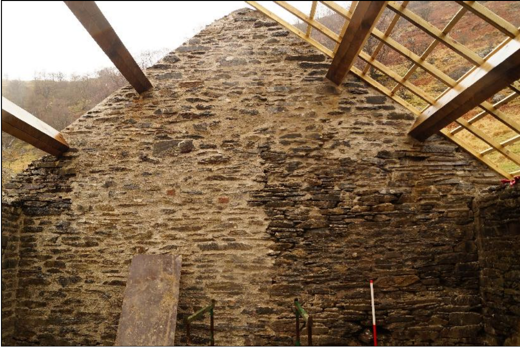
Plate 25: CEM2017_125. A view of the western gable wall of Room B. Looking west-southwest.
