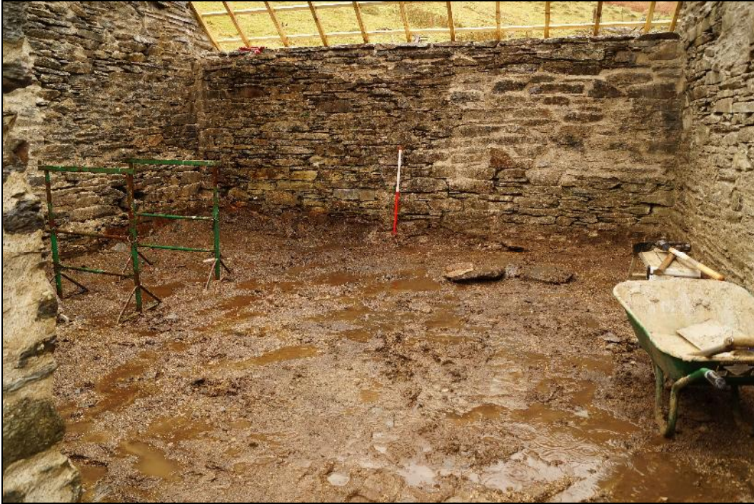
Plate 33: CEM2017_133. A view of the floor of Room B, after the removal of the mixed layer (007). This level was maintained and terram and gravel was to be laid across the interior. Looking northwest.
