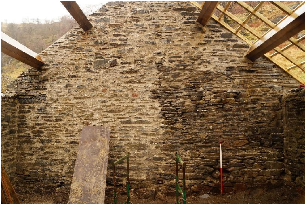
Plate 26: CEM2017_126. A view of the western gable wall of Room B, showing the base of the wall. Looking west-southwest.
