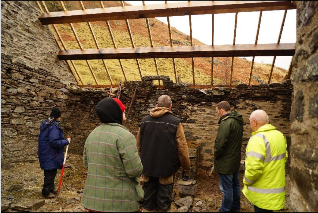
Plate 17: CEM2017_117. A view of the inside of Room A, the forge, during re-roofing. Looking north-northwest.
