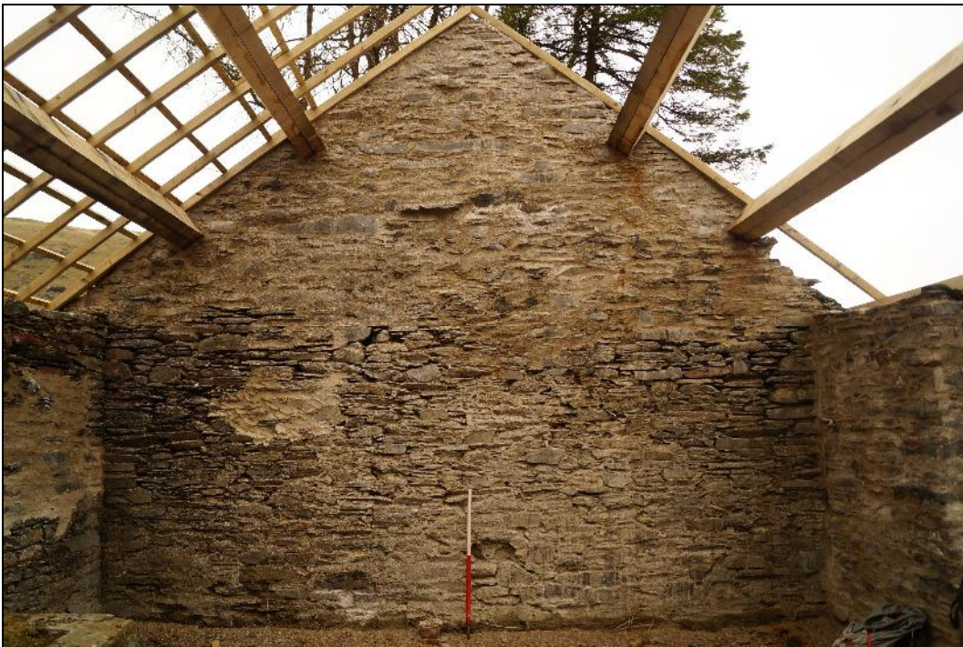
Plate 18: CEM2017_118. A view of the inside of the eastern gable wall of Room A. Looking east-northeast.
