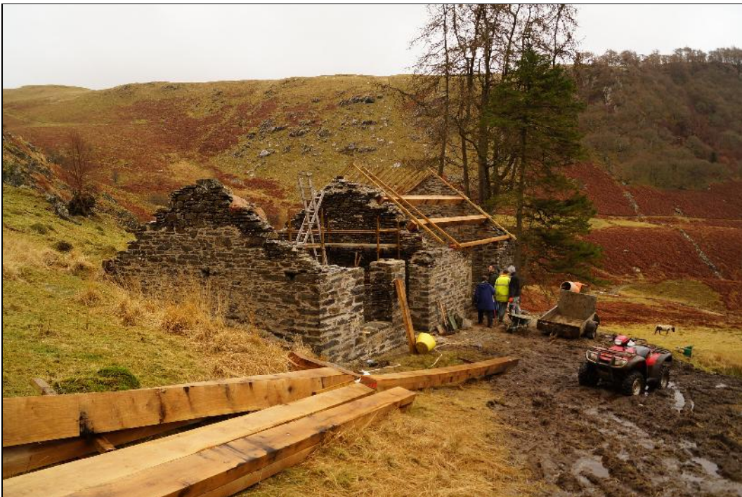
Plate 2: CEM2017_102. A view of the former mine smithy building undergoing re-roofing. Looking east-northeast.
