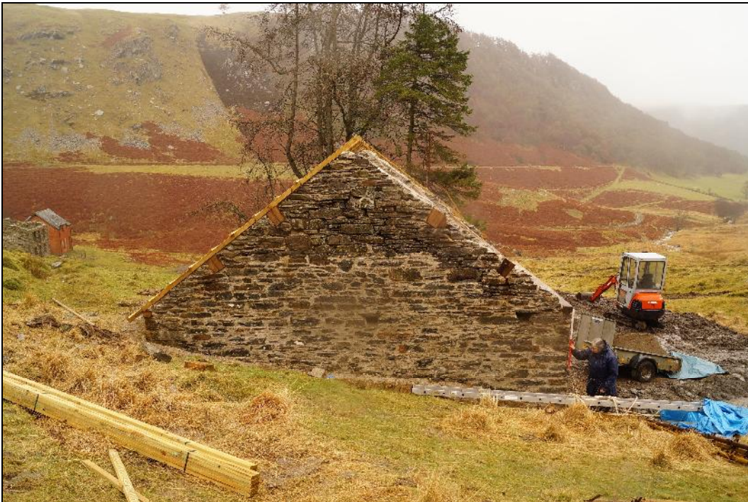
Plate 8: CEM2017_108. A view of the western gable wall of the former mine smithy. Looking east-northeast.
