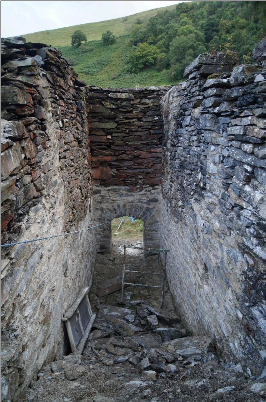
Plate 19: CEM2018_126. A view inside the wheel pit during consolidation work. Looking south-southwest.
