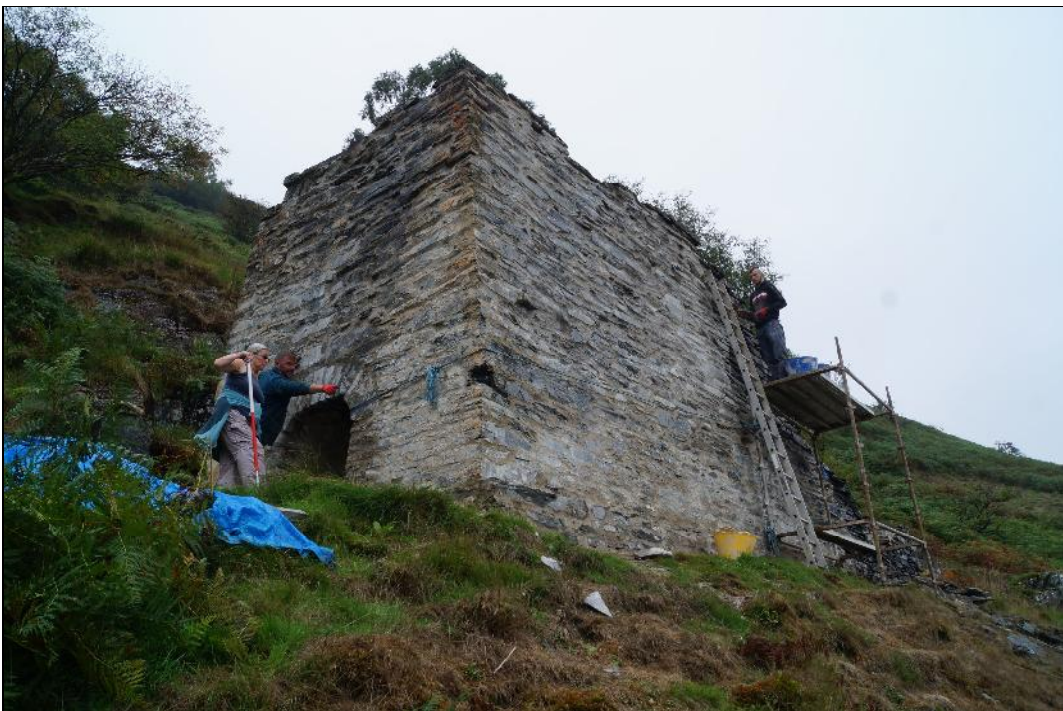
Plate 2: CEM2018_102. A view of the ruined wheel pit undergoing conservation. Looking northwest.
