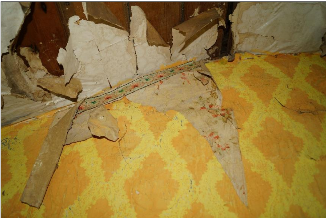
Plate 109: CYB2018_109. A view of earlier wallpaper exposed beneath the later
