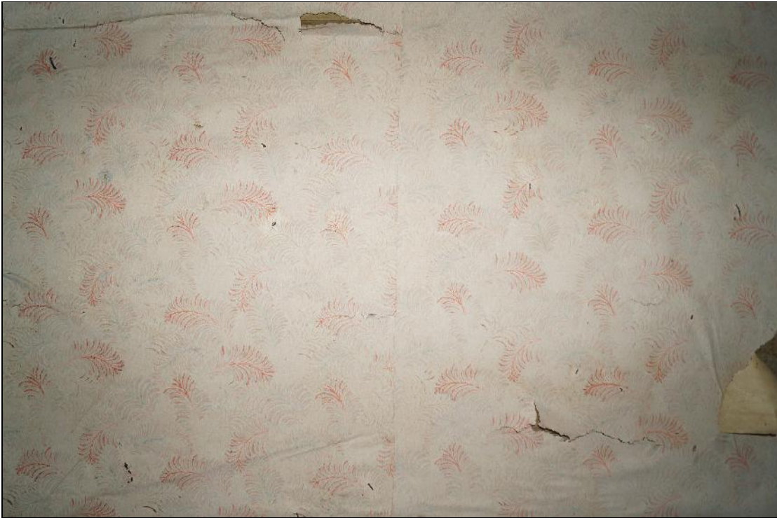
Plate 92: CYB2018_092. A view of the wallpaper on the northern wall of Room 08. Looking north-northeast.
