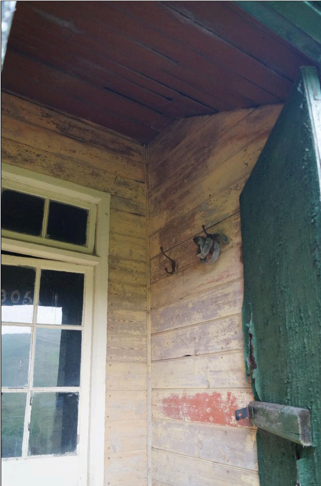
Plate 24: CYB2018_024. A view inside the porch at the front door. Looking east-northeast.
