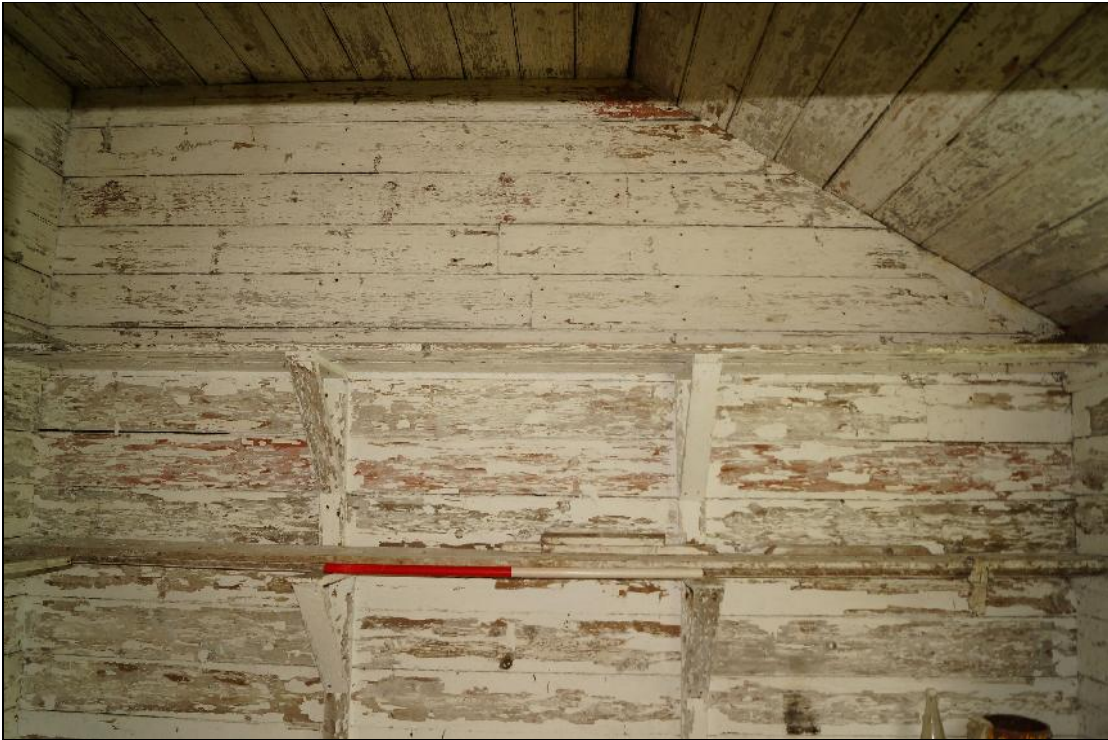
Plate 62: CYB2018_062. A view of the shelving on the west wall of Room 04 and the wooden ceiling above. Looking west-northwest.
