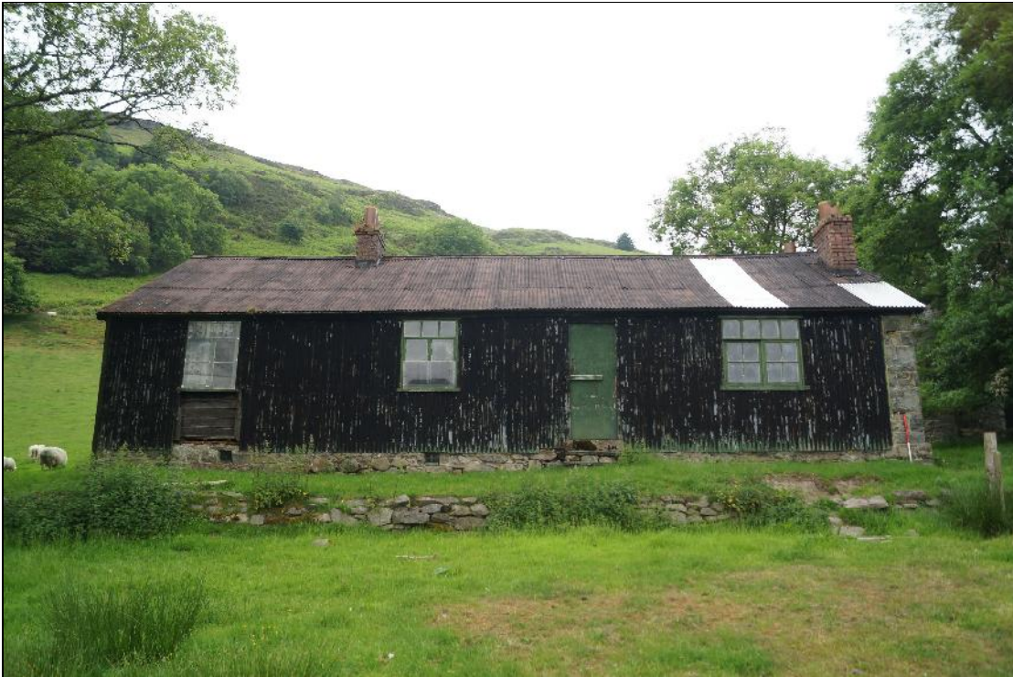
Plate 1: CYB2018_001. A view of the front of the Dam Builders' Hut. Looking north-northeast.
