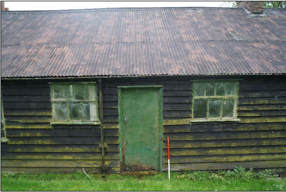
Plate 10: CYB2018_010. A view of the rear door of the Dam Builders' Hut, showing flanking windows to either side. Looking south-southwest.
