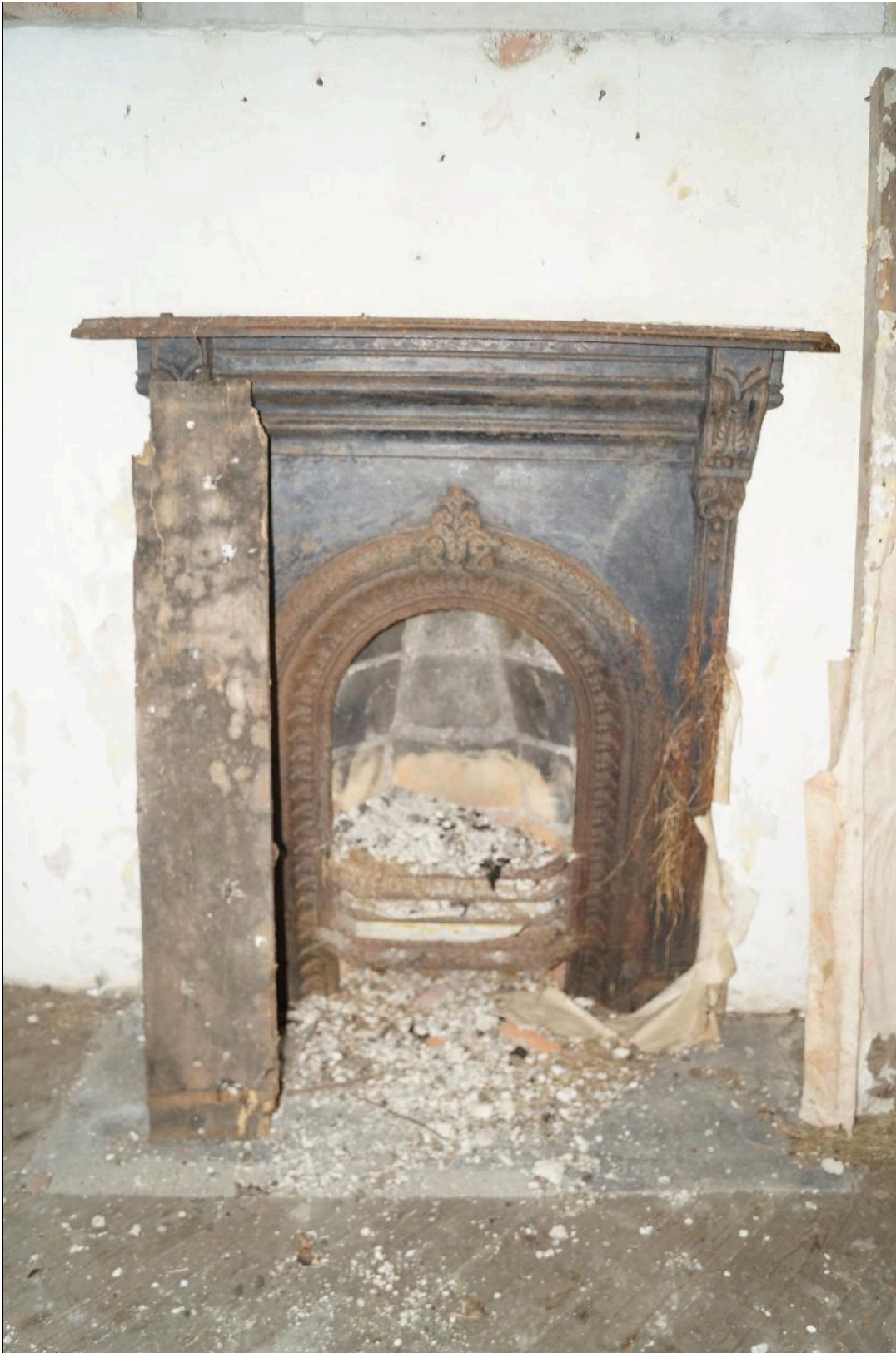
Plate 91: CYB2018_091. A view of the cast iron fireplace and hearth in Room 08. Looking east-northeast.
