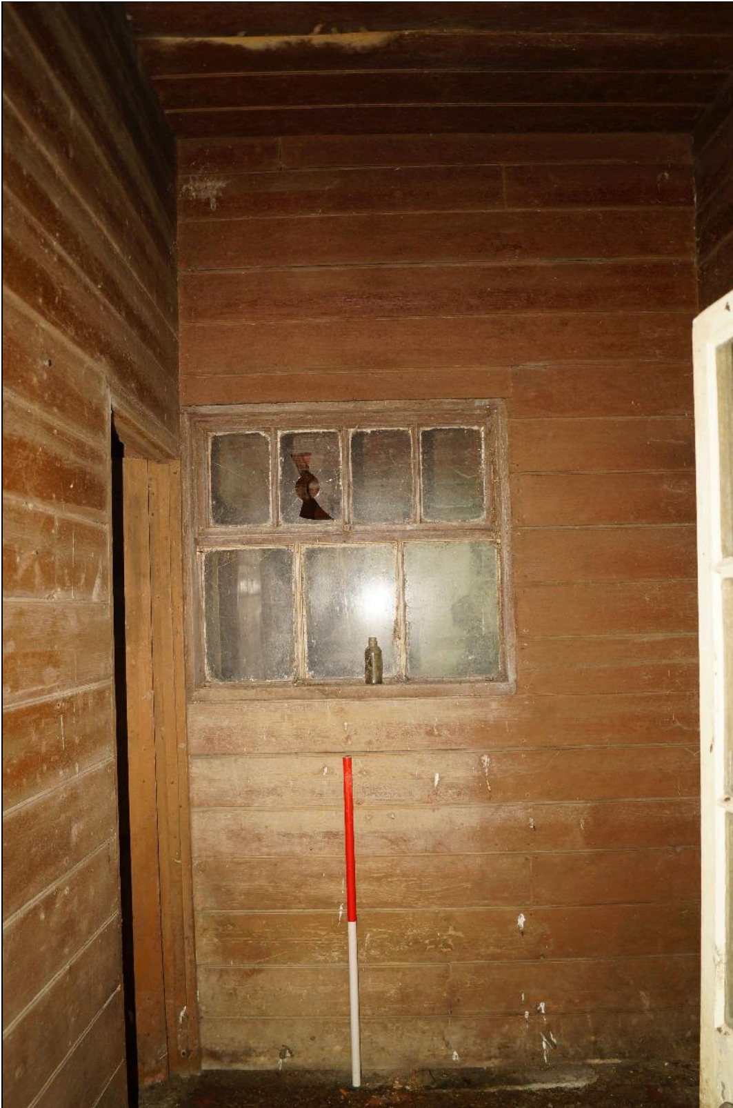
Plate 113: CYB2018_113. A view of the window between the inner porch behind the front door of the Dam Builders Hut and Room 03. Looking north-northeast.
