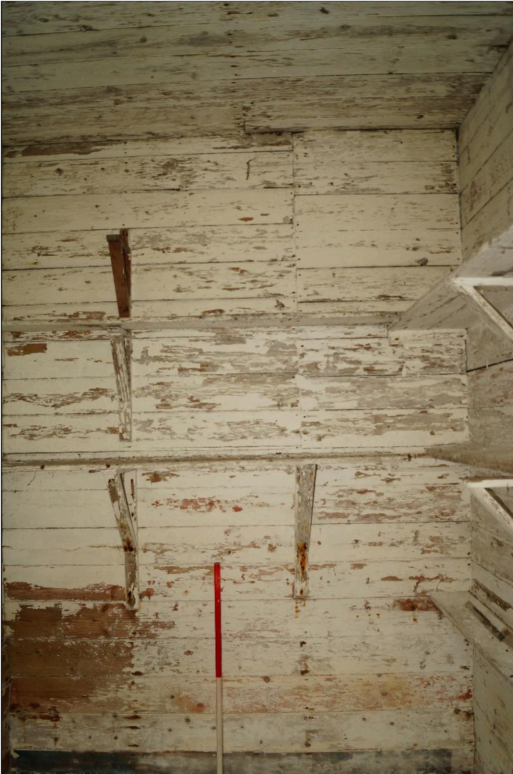
Plate 53: CYB2018_053. A view of wooden shelving on the walls inside Room 04. Looking south-southwest.
