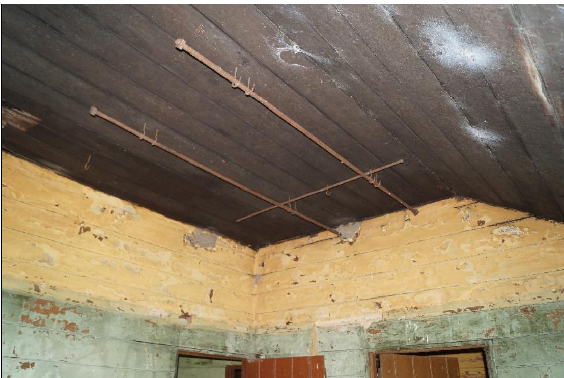
Plate 42: CYB2018_042, A view of the iron bars fixed to the ceiling of Room 02 with hooks still in place for hanging meat. Looking west-southwest.
