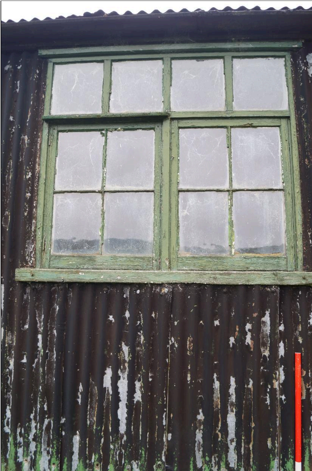
Plate 2: CYB2018_002. A view of the eastern window in the front of the Dam Builders' Hut. Looking north-northeast.
