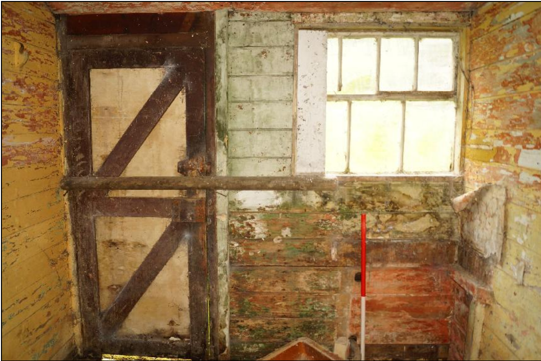
Plate 52: CYB2018_052. A view of the northern side of Room 03 showing the rear door of the hut and the window to its eastern side. Looking north-northeast.
