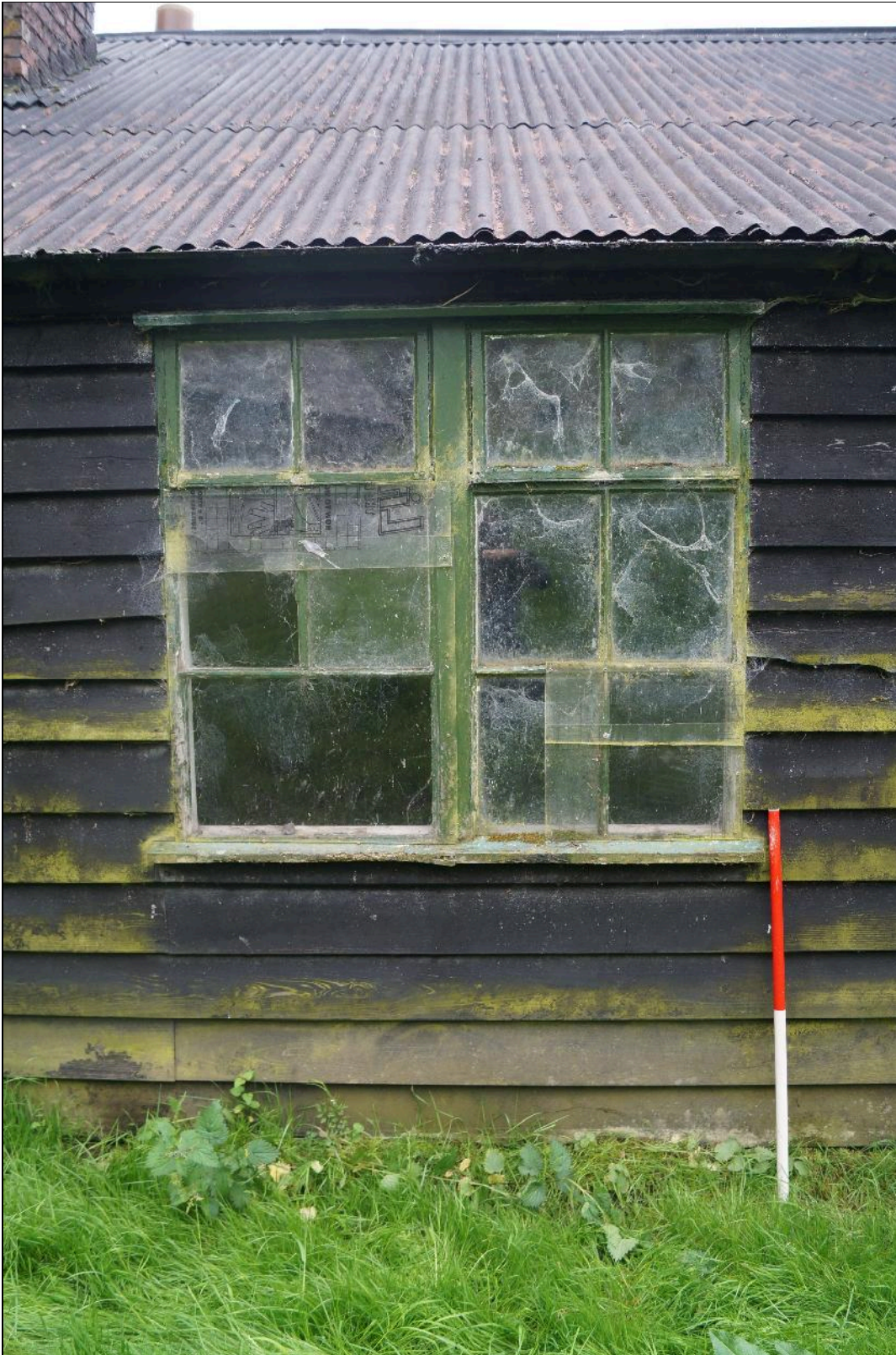
Plate 11: CYB2018_011. A view of the large eastern window to the rear of the Dam Builders' Hut. Looking south-southwest.
