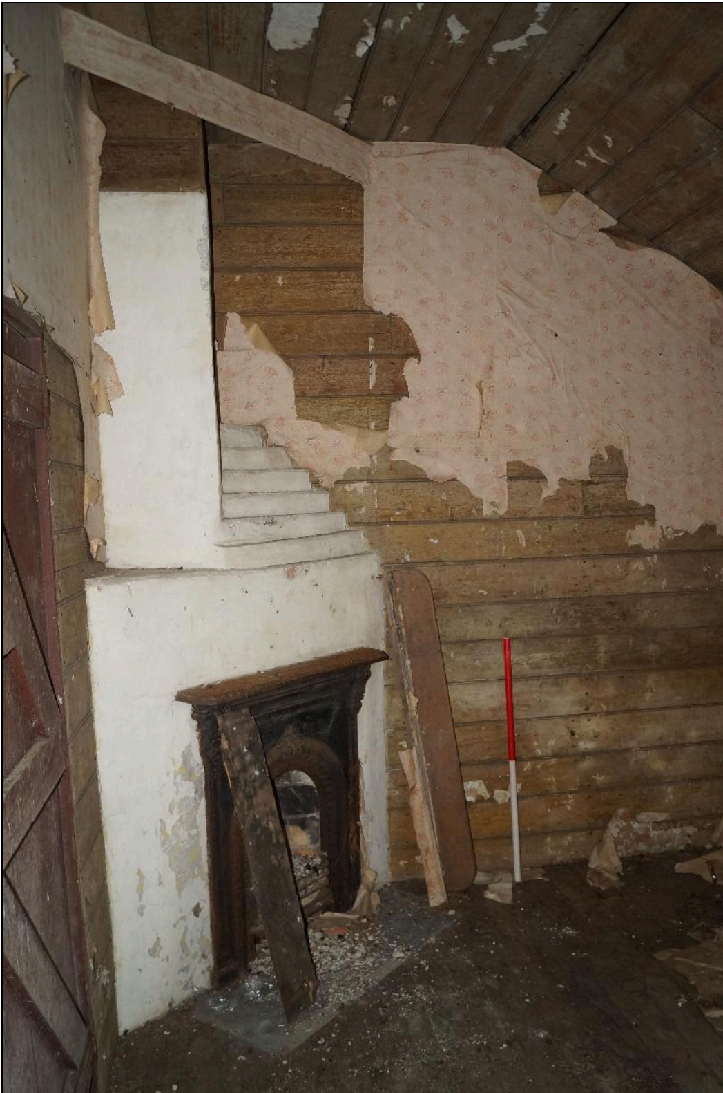
Plate 90: CYB2018_090. A view of the fireplace and eastern wall in Room 08. Looking east-southeast.
