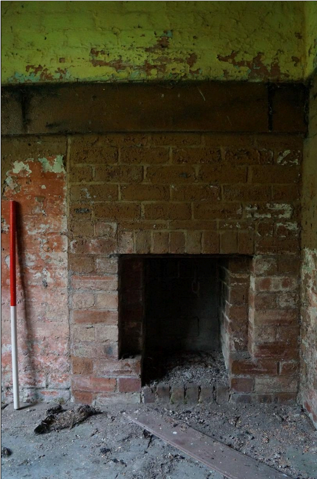
Plate 34: CYB2018_034. A view of the fireplace in Room 02. Note the flagstone floor. Looking east-southeast.
