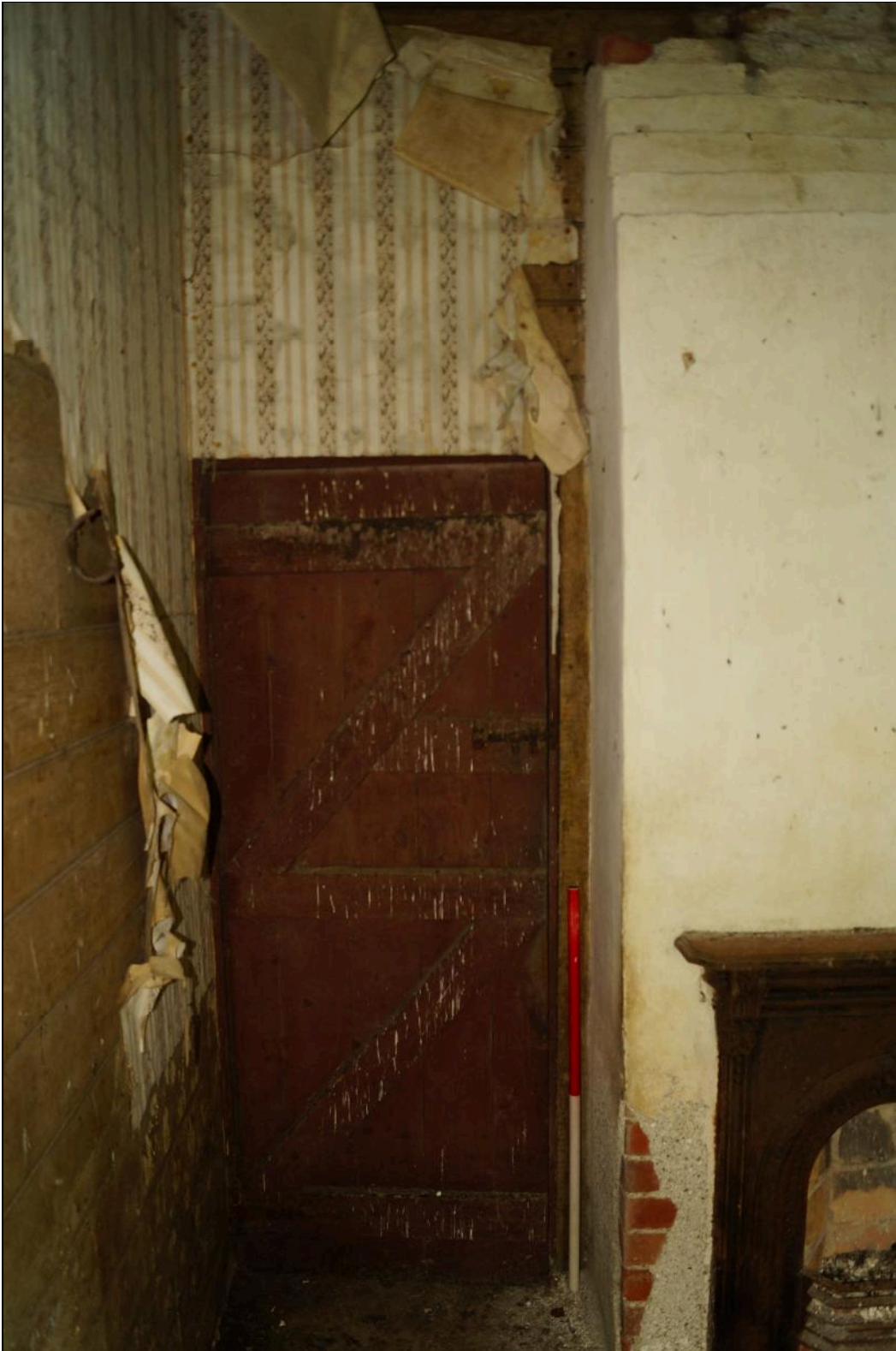
Plate 76: CYB2018_076. A view of the northern side of Room 05 showing the door exiting to the corridor (Room 07). Looking south-southwest.
