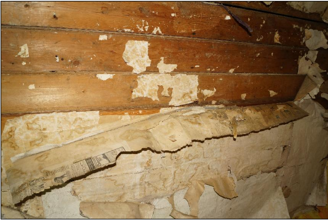
Plate 108: CYB2018_108. A view of newspaper lining on the ceiling of Room 09. Looking north-northeast.
