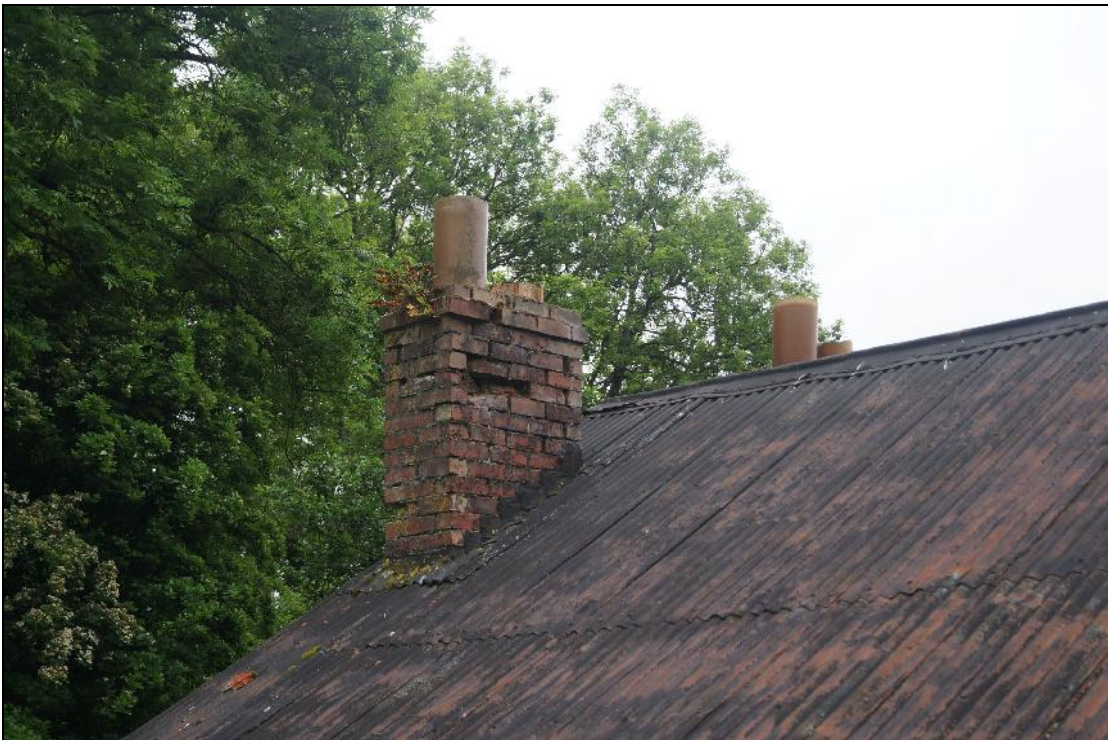
Plate 15: CYB2018_015. A view of the rear eastern chimney of the Dam Builders' Hut. Looking south-southeast.
