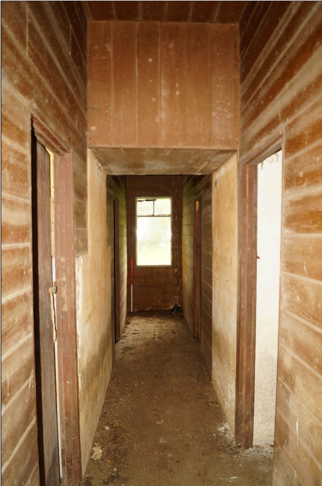
Plate 63: CYB2018_063. A view along the central corridor Room 07. The doors to rooms 09 and 08 are to the left and Rooms 05 and 06 to the right. Looking west-northwest.
