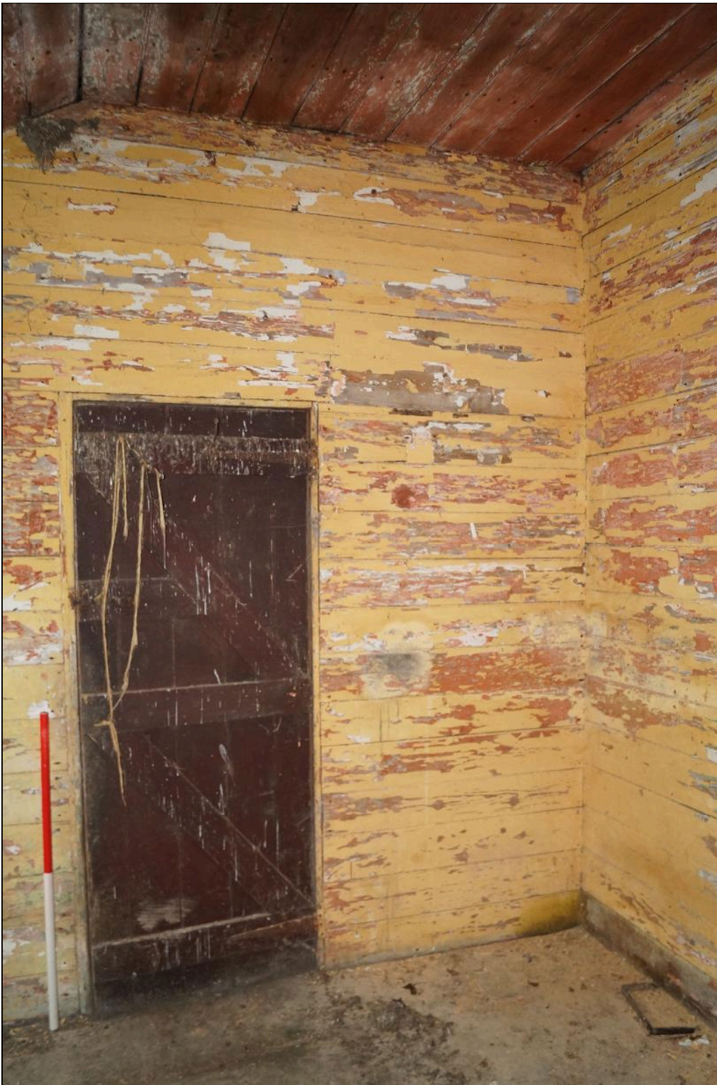
Plate 49: CYB2018_049. A view of the doorway leading from Room 03 into Room 02, viewed from the doorway between Room 03 and Room 04. Looking southeast.
