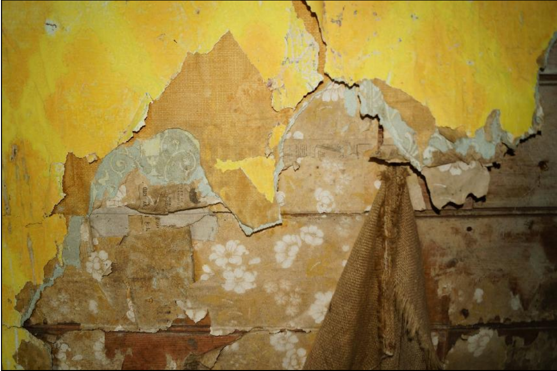
Plate 112: CYB2018_112. A view of several layers of overlapping wallpaper and newspaper lining visible in the northern wall of Room 09. Looking north-northeast.
