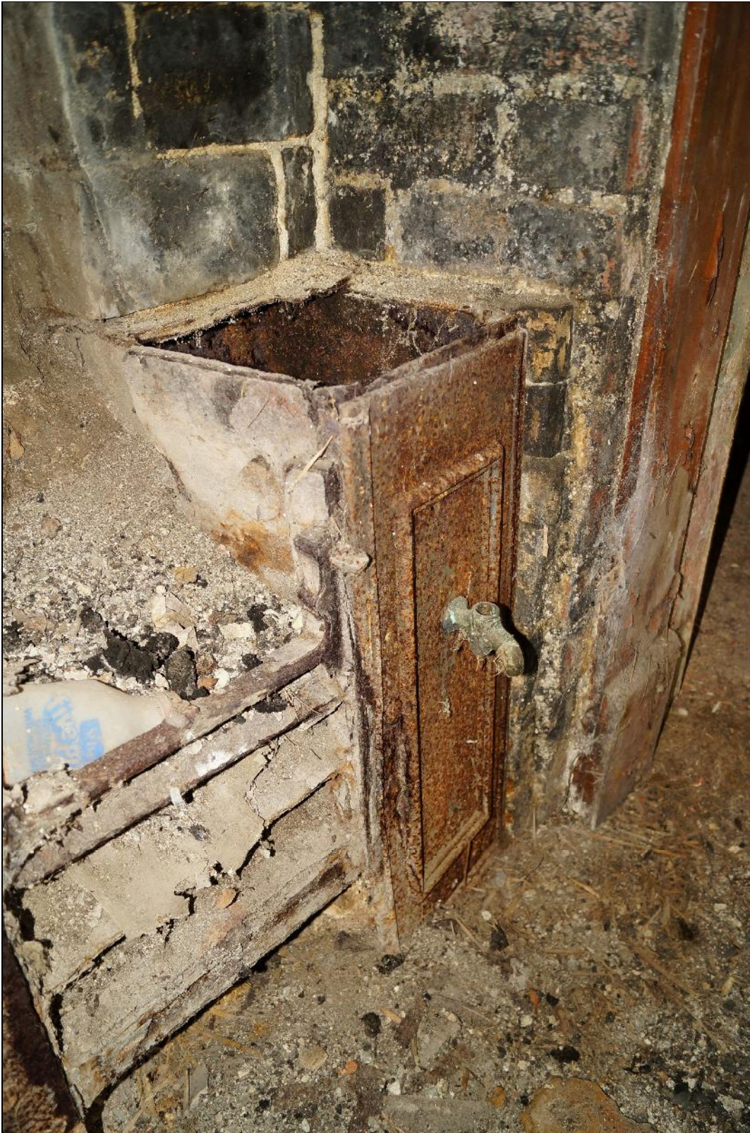
Plate 31: CYB2018_031. A view of the water heating tank built into the fireplace of Room 01. Looking south.
