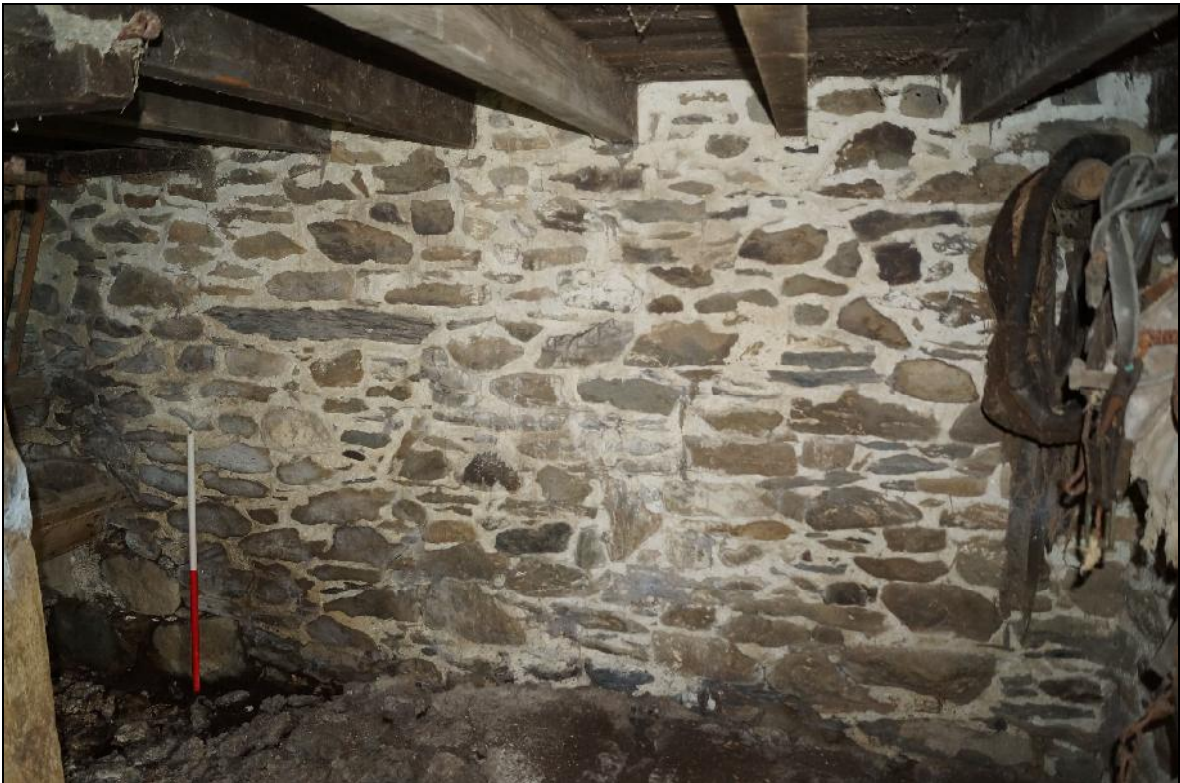
Plate 28: CYD2018_028, an internal view of the southern wall of the stable, looking south-southeast.
