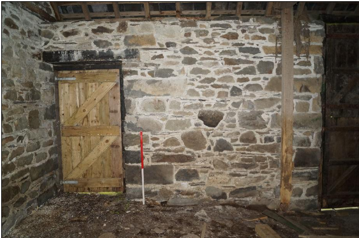
Plate 132: CYD2018_132, an interior view of the barn, looking east towards the closed single door.
