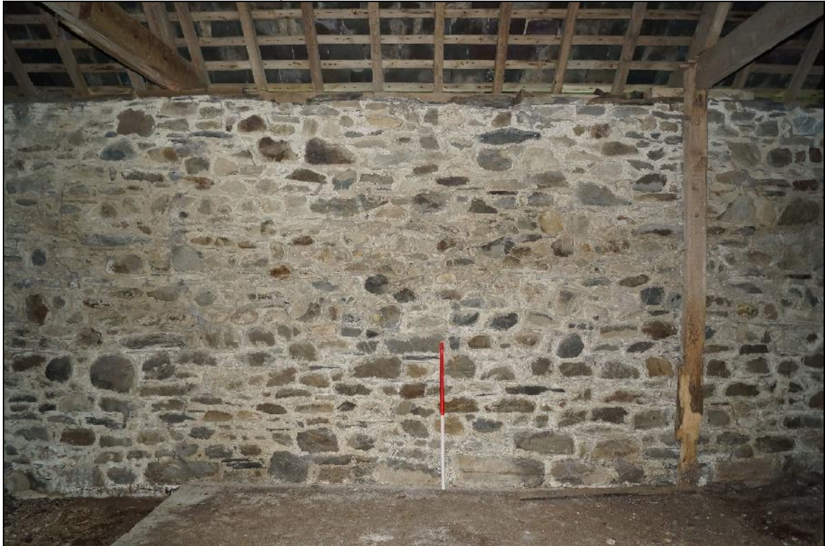
Plate 125: CYD2018_125, an interior view of the barn, looking west towards the central portion of the west wall.
