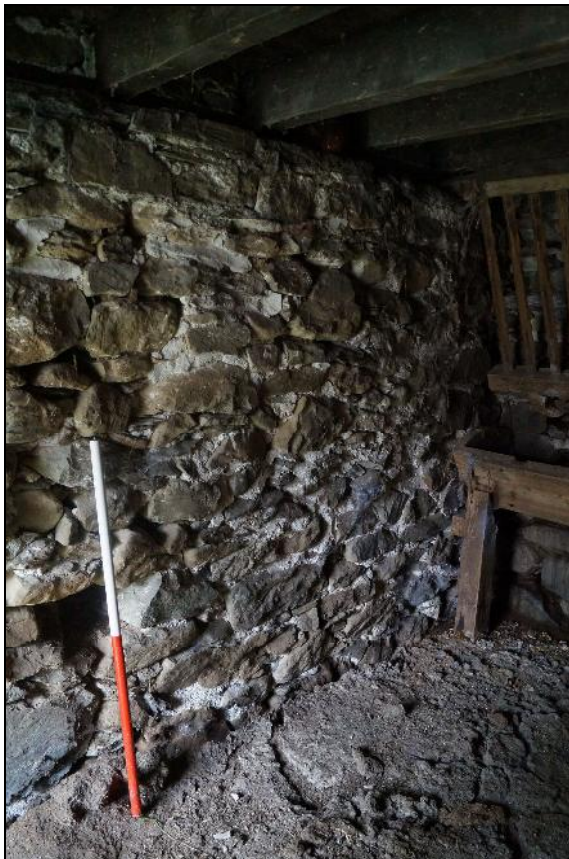
Plate 32: CYD2018_032, an internal view of the stable, showing the eastern end of the northern wall, looking north-northeast.
