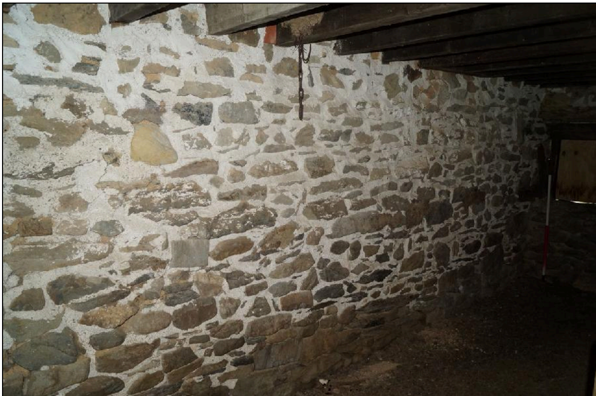
Plate 62: CYD2018_062, internal view of the cowshed, showing the southern wall and looking southwest.
