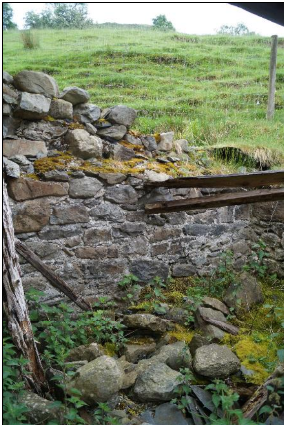
Plate 36: CYD2018_036, a view of the ruined lean-to extension at the southern end of the stable and cartshed building, looking south-southeast.
