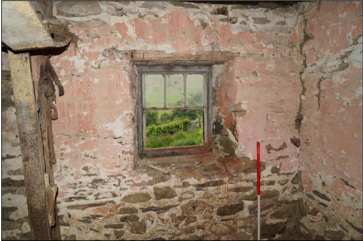
Plate 83: CYD2018_083, an interior view of the western wall of the "parlour", looking west-southwest.
