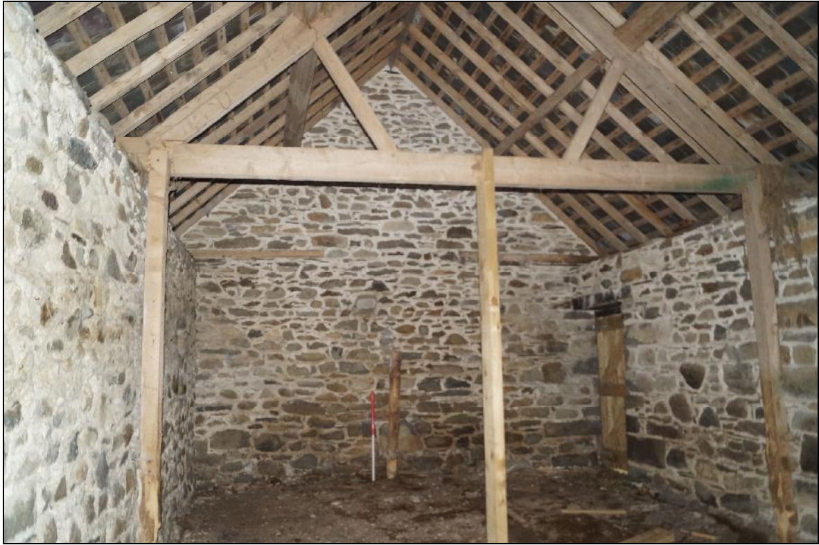
Plate 129: CYD2018_129, an interior view of the barn, looking north-northeast towards the gable wall. Note the modern roof and supporting timbers.
