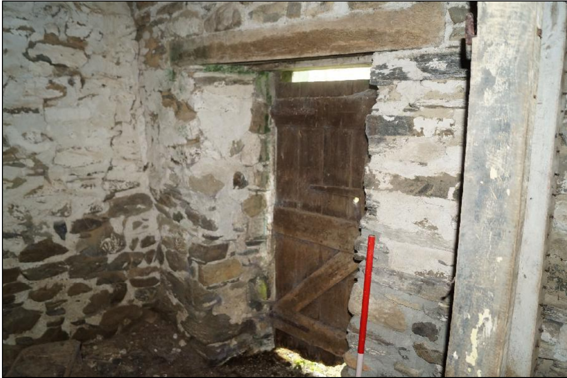
Plate 71: CYD2018_071, the doorway in the eastern wall of the "dairy", looking north.
