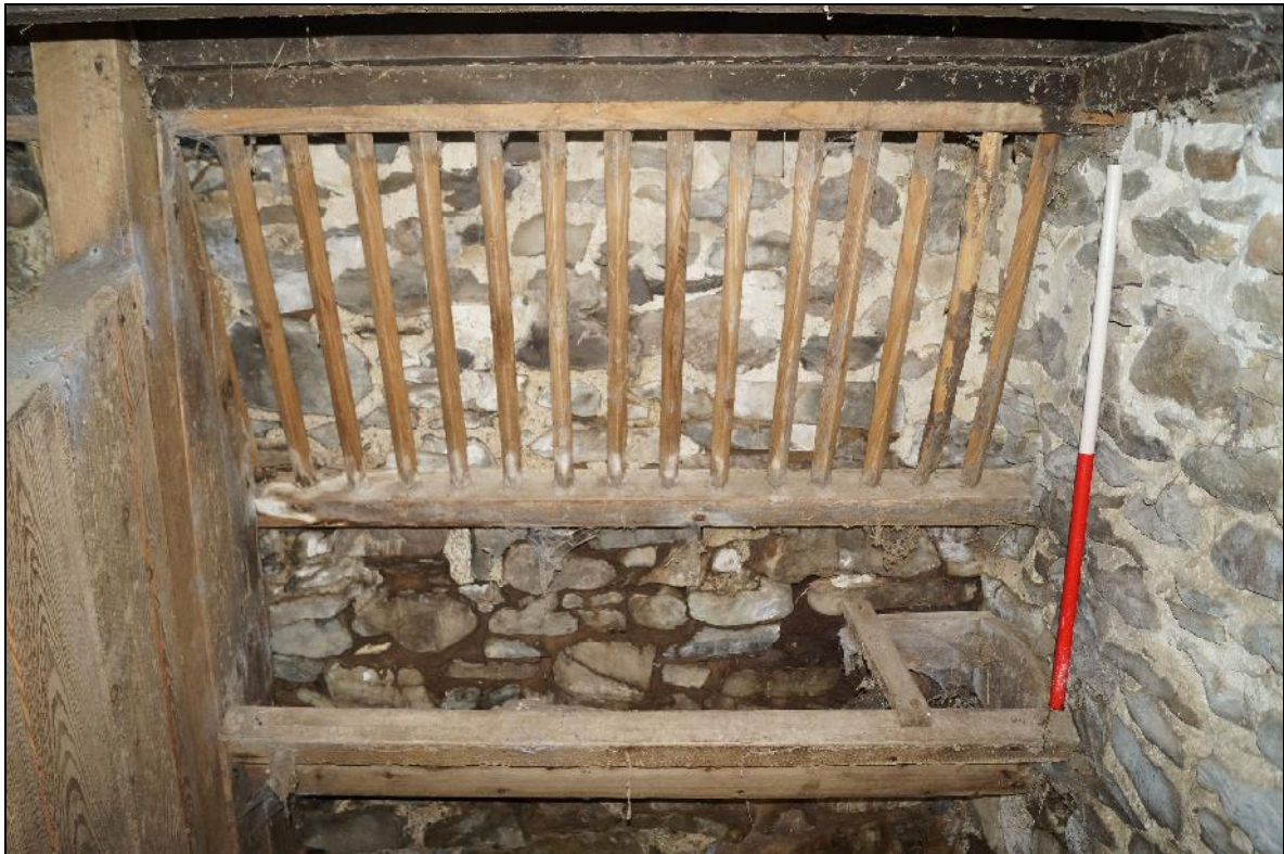
Plate 24: CYD2018_024, an internal view of the stable, showing detail of the southern feeding stall, looking east-northeast.
