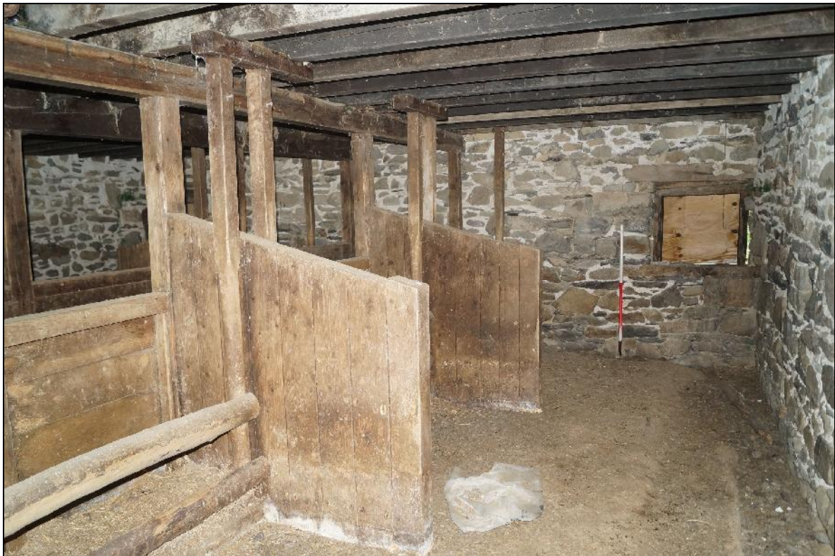
Plate 46: CYD2018_046, internal view of the cowshed, showing the feeding stalls at the northern end of the cowshed and looking southwest. A pitching door is seen on the far wall.
