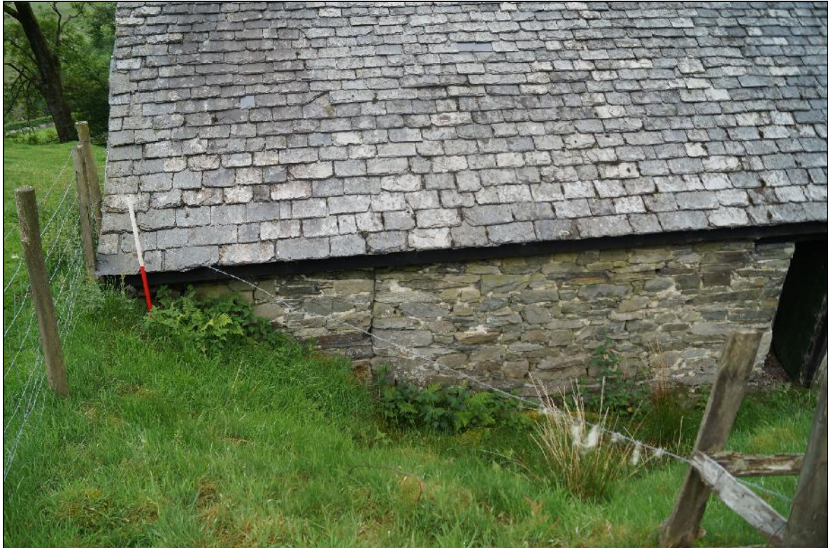
Plate 43: CYD2018_043, external view of the southern end of the house and cowshed building, looking west-southwest, showing rip joint said to represent an original doorway (see Plates 90 & 91 for internal views).
