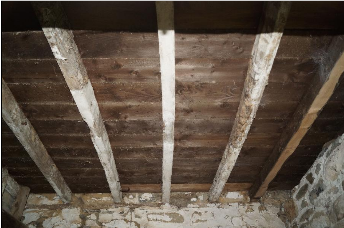
Plate 77: CYD2018_077, a view of the beams in the ceiling of the "dairy", which include modern, machine-sawn timber (furthest to right) as well as at least one hand-cut beam (second beam to right), looking north-northwest.
