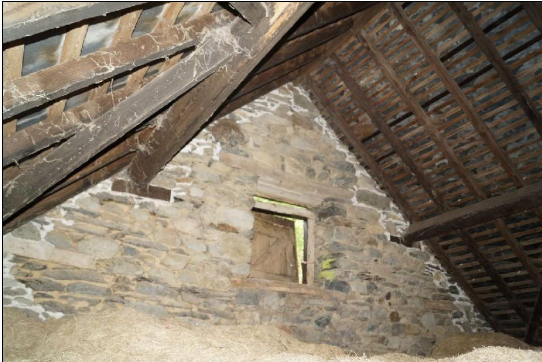
Plate 55: CYD2018_055, internal view of the access to the cowshed hayloft in the northern gable wall, viewed through a hatch in the cowshed ceiling, looking north.
