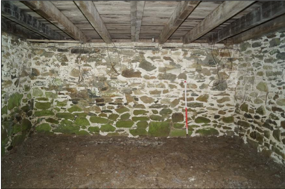
Plate 17: CYD2018_017, internal view of the southern wall of the cartshed, looking south-southeast.
