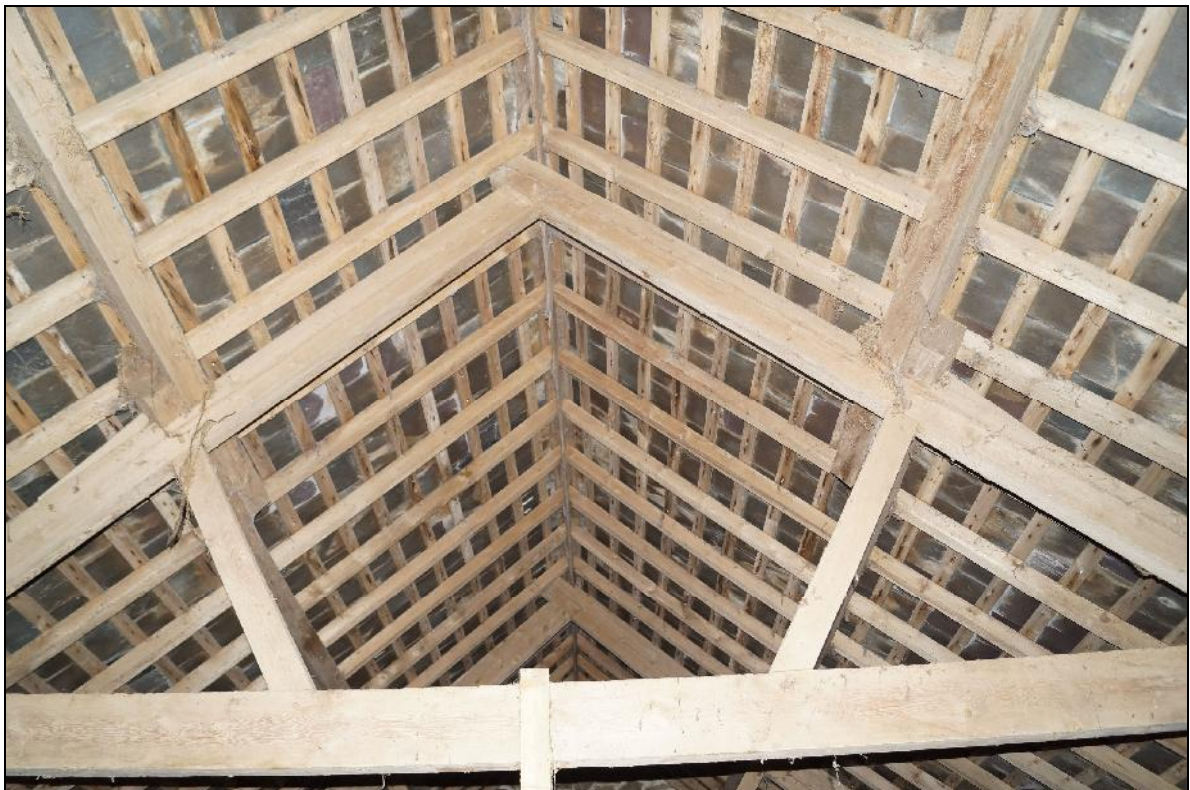
Plate 136: CYD2018_135, an interior view of the barn roof, which is a modern construction. Roofing nails have been used to fix the slates, whereas as wooden pegs were used to re-roof the house and cowshed. Looking north.
