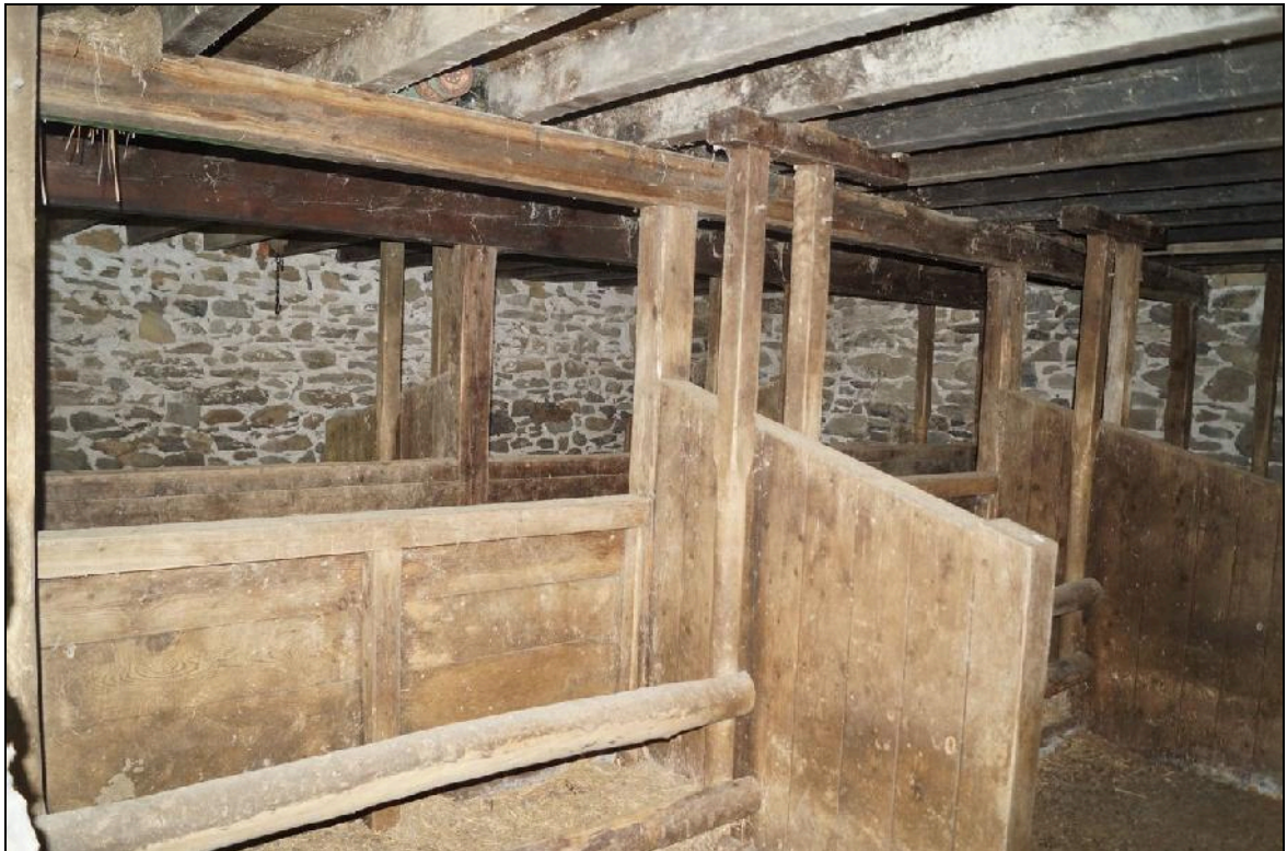
Plate 66: CYD2018_066, internal view of the cowshed, showing the northern feeding stalls, looking south-southwest.
