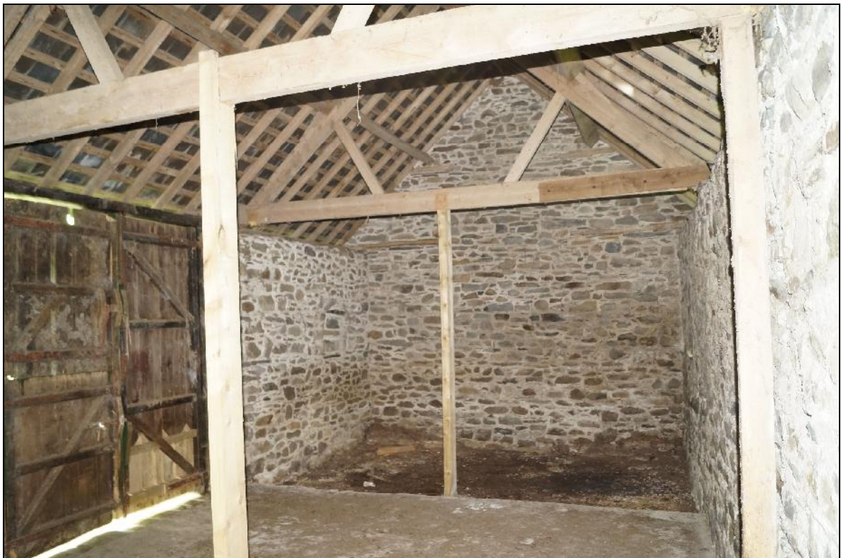
Plate 134: CYD2018_133, an interior view of the barn, looking south-southeast towards the gable wall. Note the modern roof and supporting timbers
