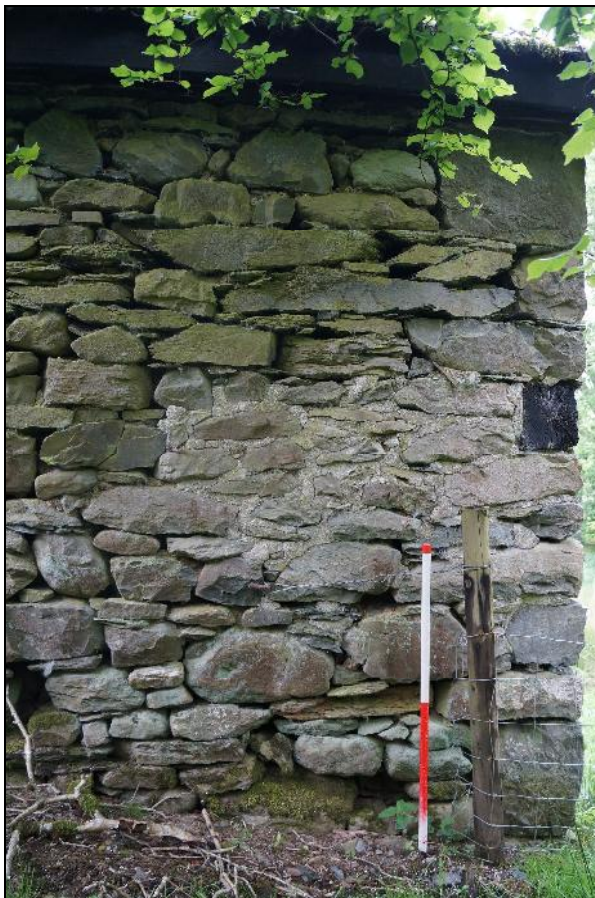
Plate 14: CYD2018_014, external view of the northern end of the eastern wall of the cartshed and stable building, looking west-southwest.
