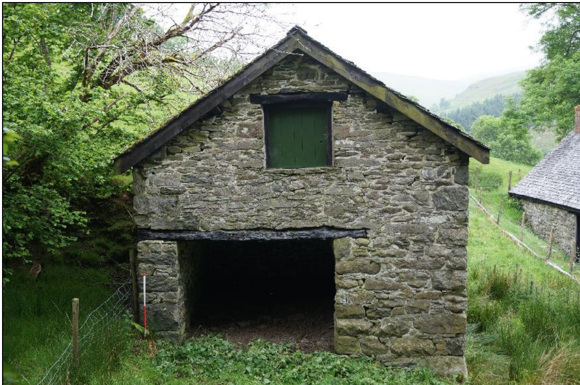
Plate 12: CYD2018_012, external view of the stable and cartshed building looking south-southeast, showing the cartshed entrance and hayloft door above.
