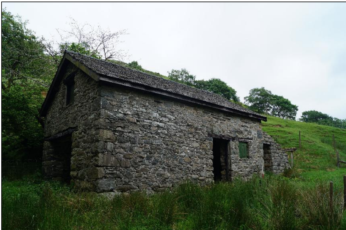
Plate 4: CYD2018_004, external view of the stable and cartshed building looking east-southeast. Note cartshed entrance, with hayloft door above, to the left of the image.
