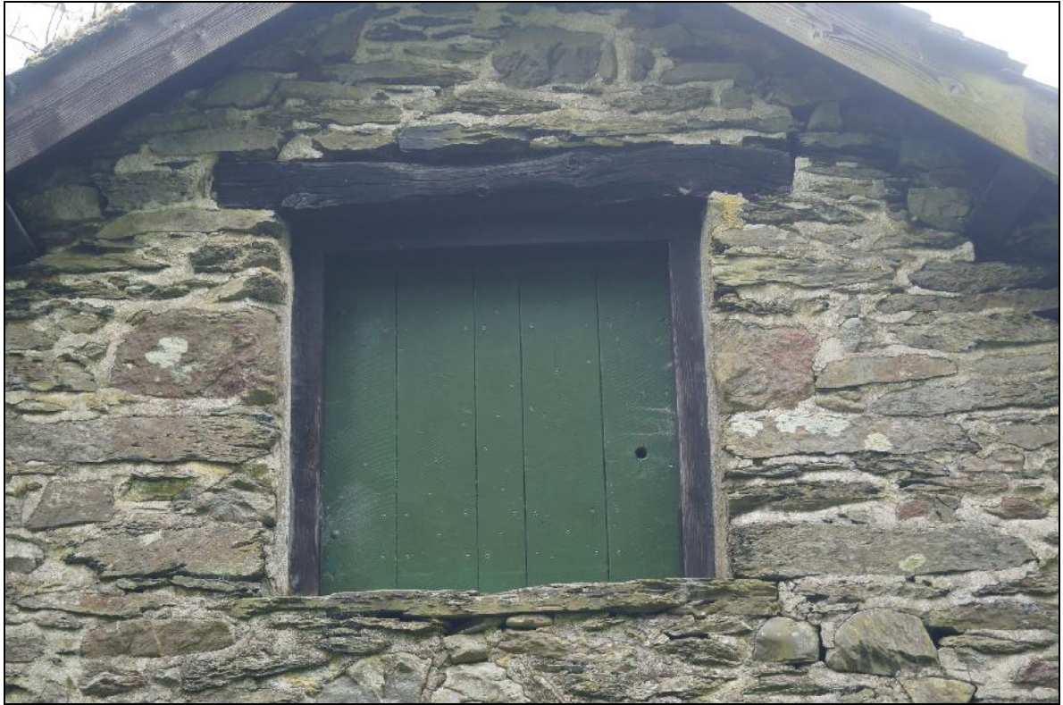
Plate 21: CYD2018_021, external view of the stable and cartshed building looking south-southeast, showing the hayloft door.
