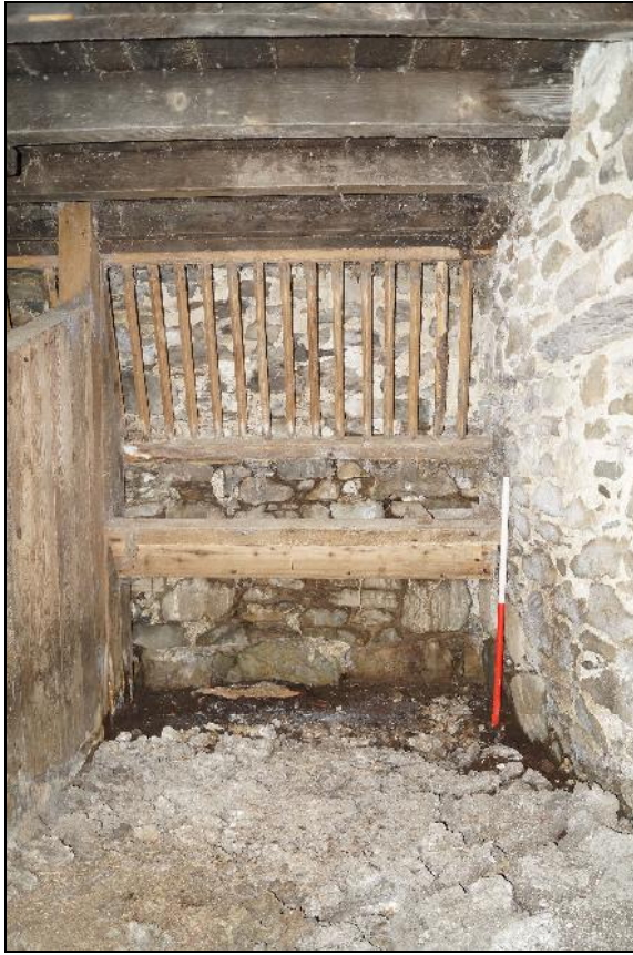
Plate 23: CYD2018_023, an internal view of the stable, showing the southern feeding stall, looking east-northeast.
