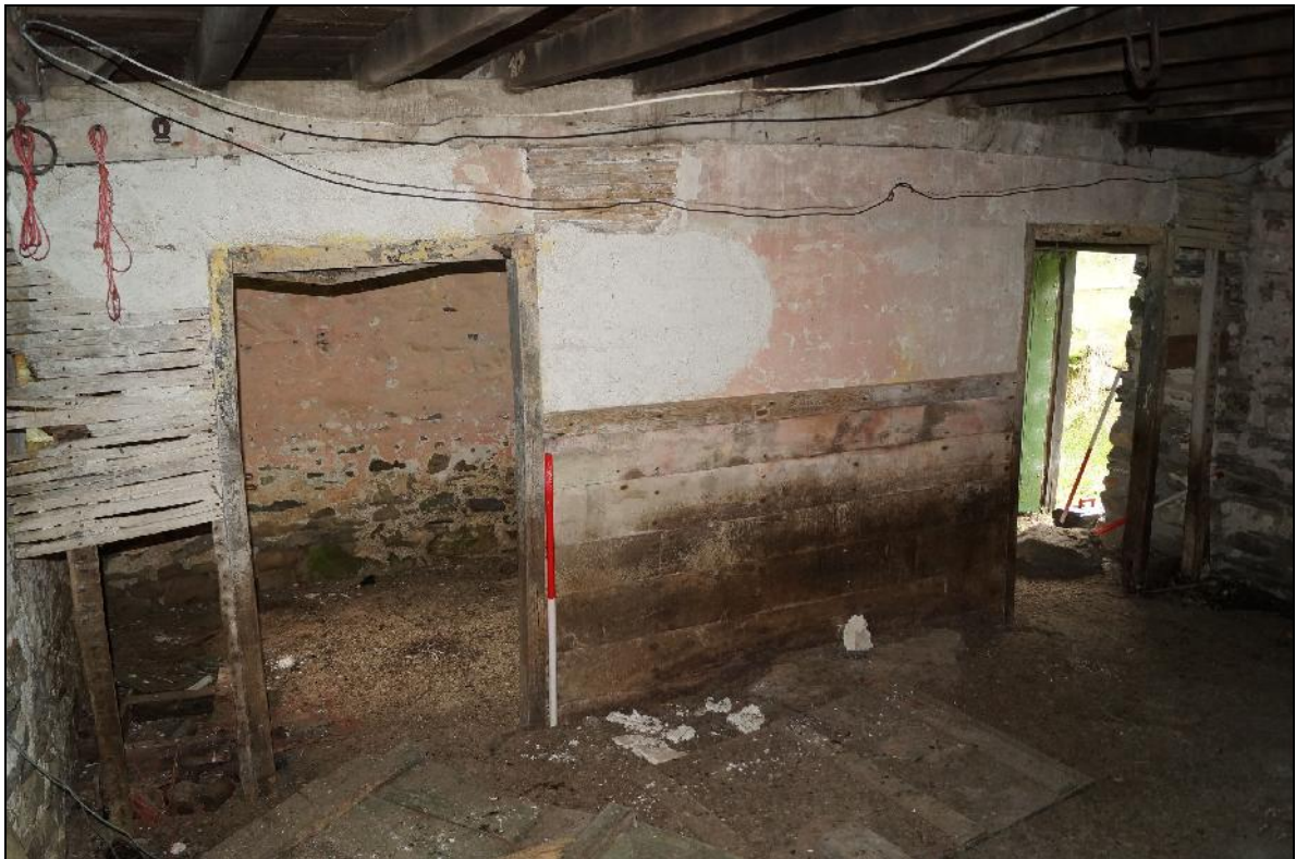
Plate 86: CYD2018_086, an interior view of the kitchen, looking north, showing the doorways leading into the parlour (left) and "dairy" (right).
