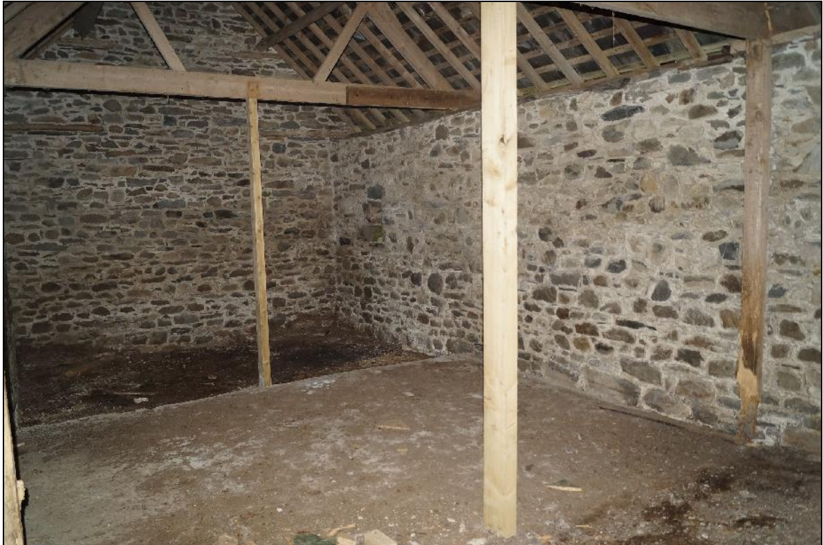
Plate 133: CYD2018_132, an interior view of the barn, looking south-southwest towards the gable wall. Note the modern roof and supporting timbers
