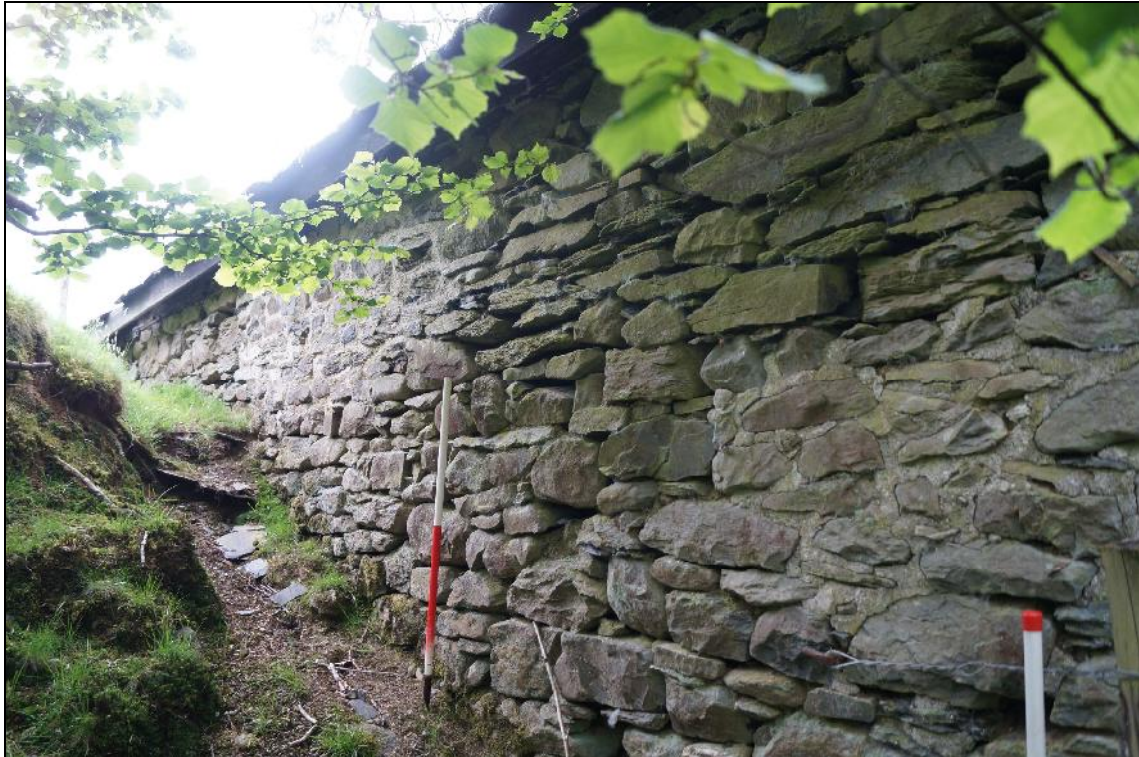
Plate 15: CYD2018_015, external view of the eastern wall of the cartshed and stable building, looking south-southwest.
