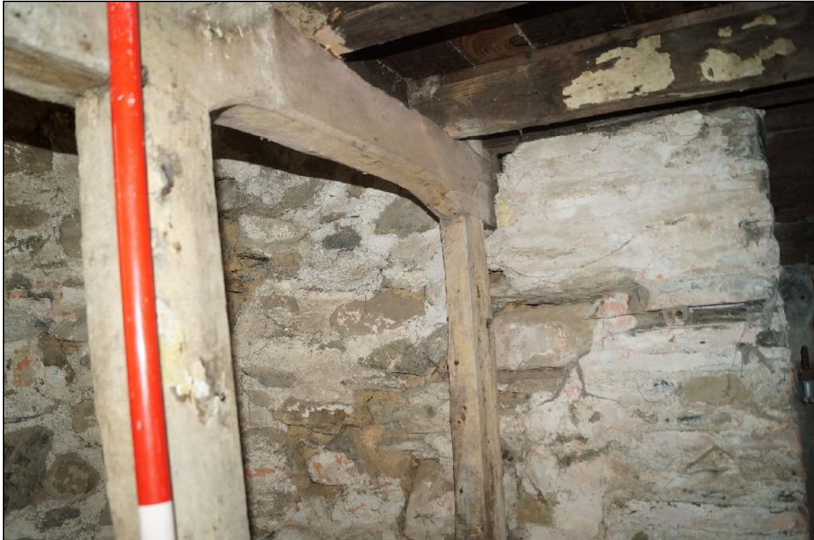
Plate 99: CYD2018_099, a view of the moulded doorframe around the doorway leading from the kitchen to the loft stairs, looking south-southwest.
