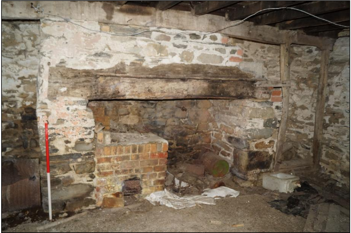
Plate 93: CYD2018_093, an interior view of the fireplace in the kitchen, looking south. The brick insert was the housing for a water boiler.
