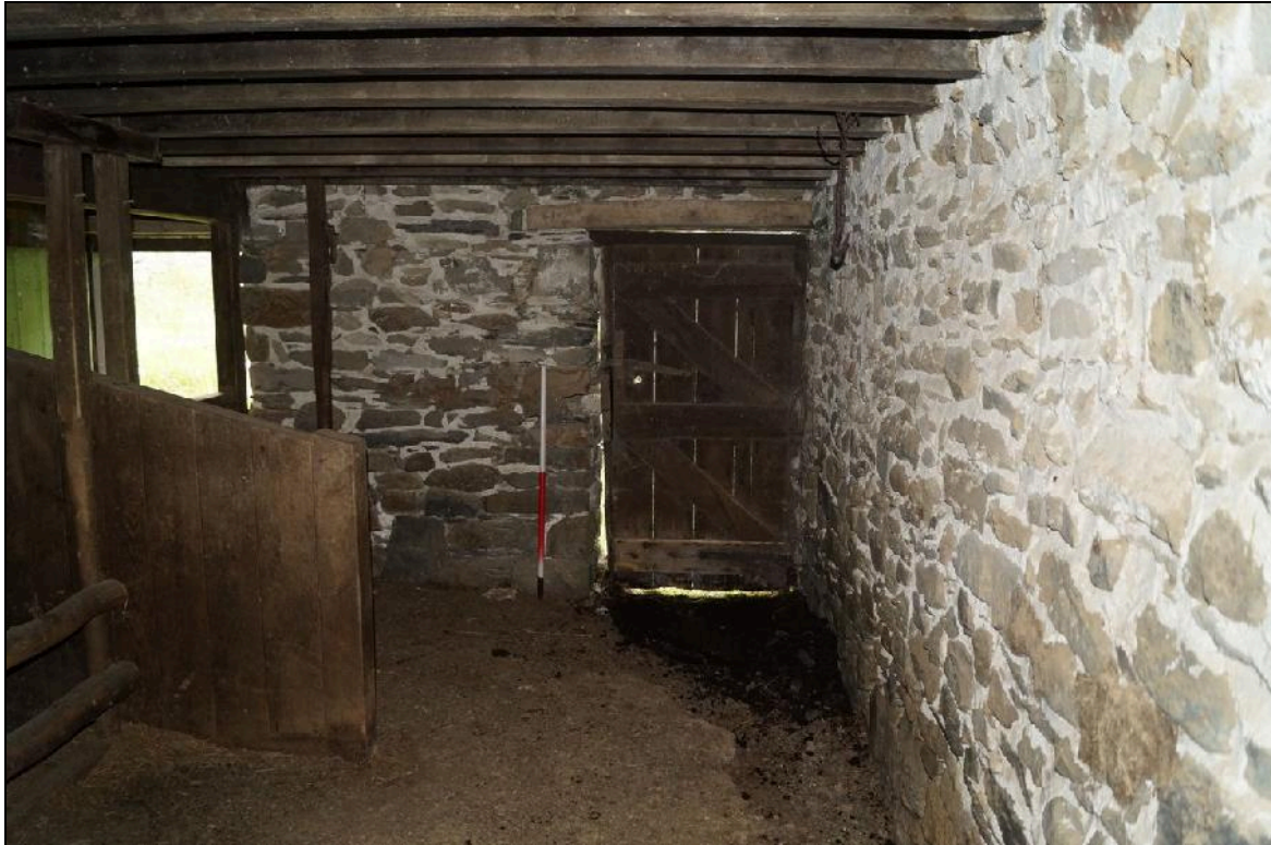
Plate 61: CYD2018_061, internal view of the cowshed, showing the feeding stalls at the southern end of the cowshed with the doorway in the east wall, looking east-northeast.
