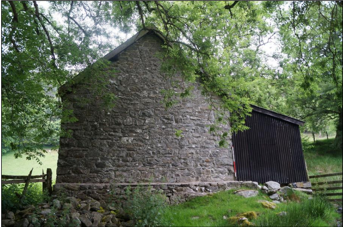
Plate 115: CYD2018_115, an external view of the southern gable wall of the barn at Cwmclyd, looking north.
