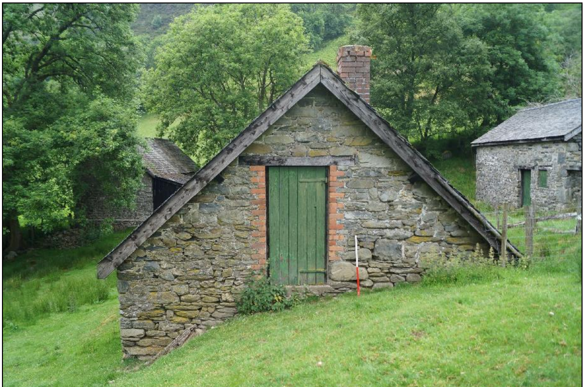
Plate 40: CYD2018_040, an external view of the south wall of the house and cowshed building, looking north-northwest.
