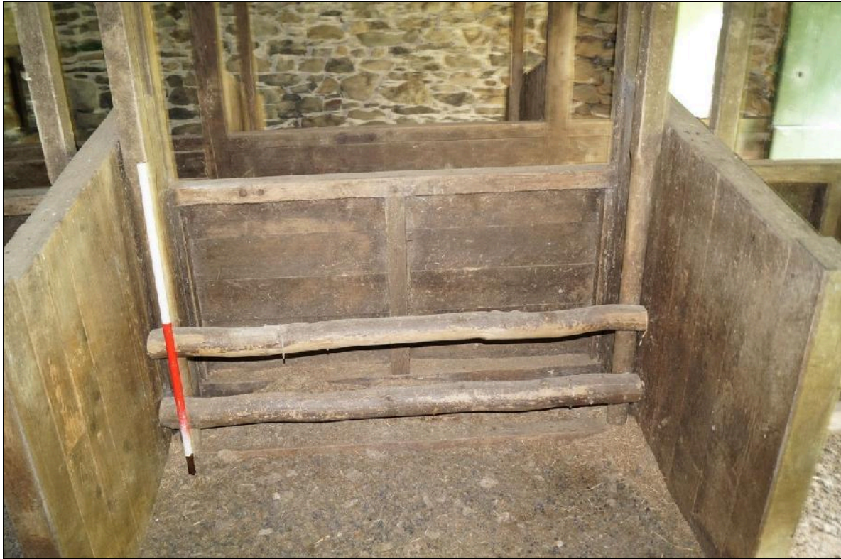
Plate 59: CYD2018_059, internal view of the cowshed, showing the central feeding stall at the southern end of the cowshed and looking north-northwest.
