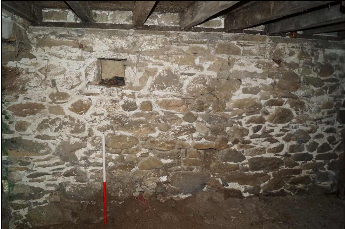
Plate 31: CYD2018_031, an internal view of the stable, showing the northern wall, looking north-northwest.
