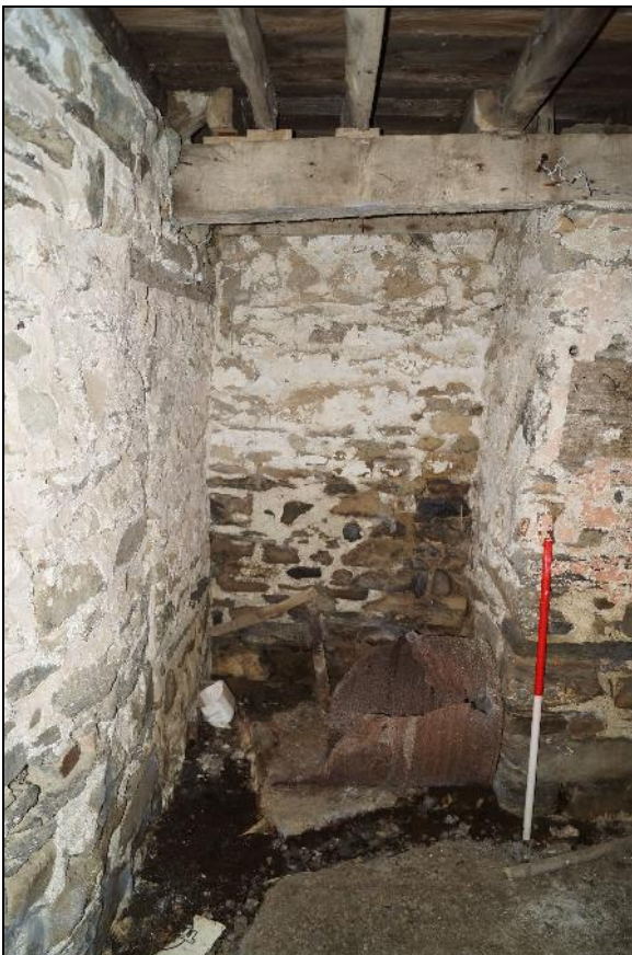
Plate 92: CYD2018_092, an interior view of the southeastern corner of the kitchen, looking southeast, showing an alcove inside the apparent blocked up doorway.
