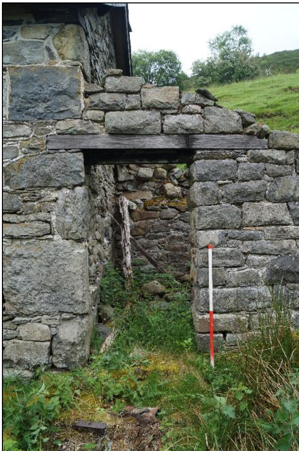
Plate 10: CYD2018_010, external view of the doorway of the now roofless lean-to extension at the southern end of the stable looking east-northeast.
