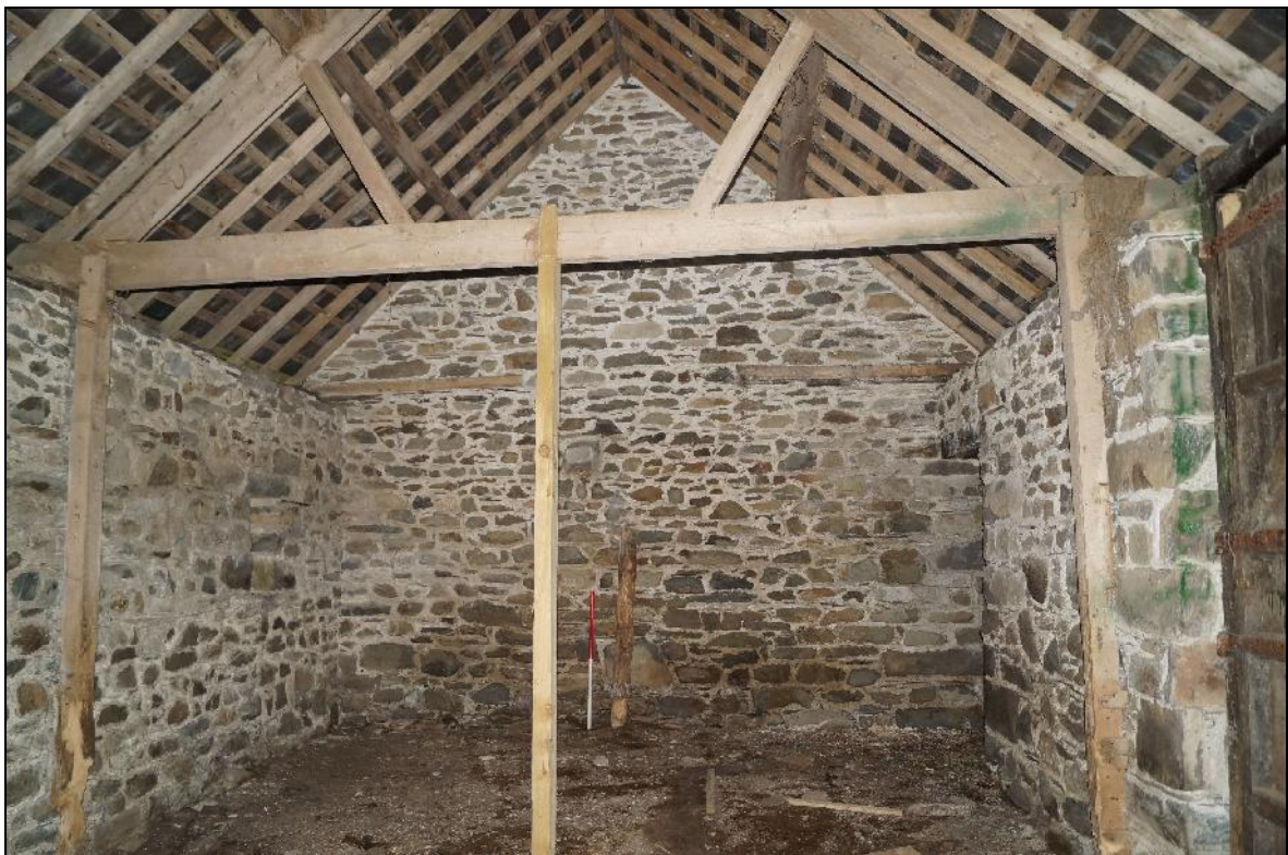
Plate 128: CYD2018_128, an interior view of the barn, looking north-northwest towards the gable wall. Note the modern roof and supporting timbers.
