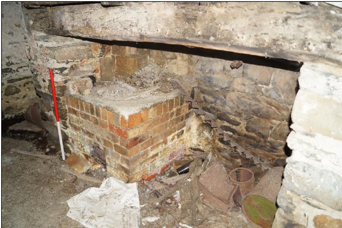
Plate 96: CYD2018_096, a close-up of the fireplace and boiler housing in the kitchen, looking southeast.
