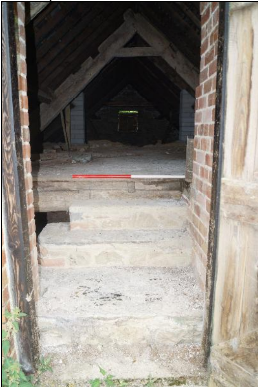
Plate 104: CYD2018_104, a view through the loft door in the southern gable wall of the house, which also gave access to the steps down to the kitchen, looking north-northwest.
