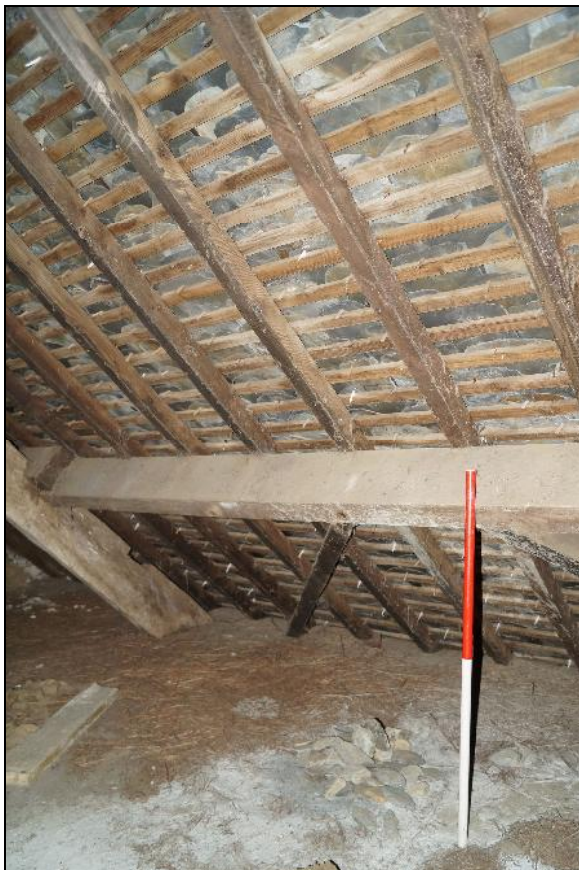
Plate 106: CYD2018_106, a view of the modern roof from inside the loft, looking northeast.
