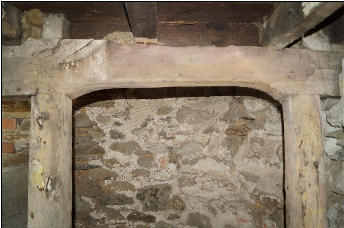
Plate 100: CYD2018_100, a view of the moulded doorframe around the doorway leading from the kitchen to the loft stairs, looking south-southeast.
