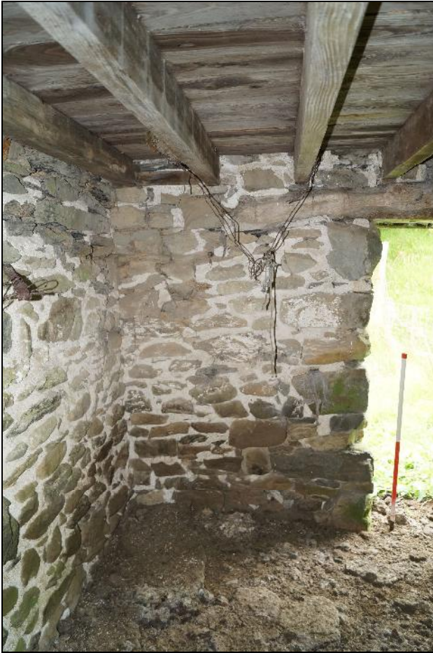
Plate 19: CYD2018_019, internal view of the northern side of the cartshed, looking north-northwest.
