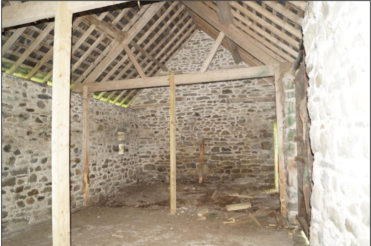
Plate 135: CYD2018_134, an interior view of the barn, looking north-northwest towards the gable wall. Note the modern roof and supporting timbers
