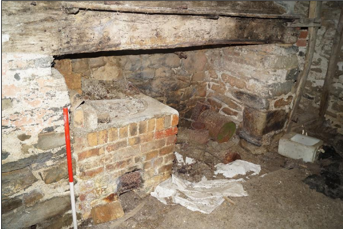
Plate 95: CYD2018_095, a close-up of the fireplace and boiler housing in the kitchen, looking south.
