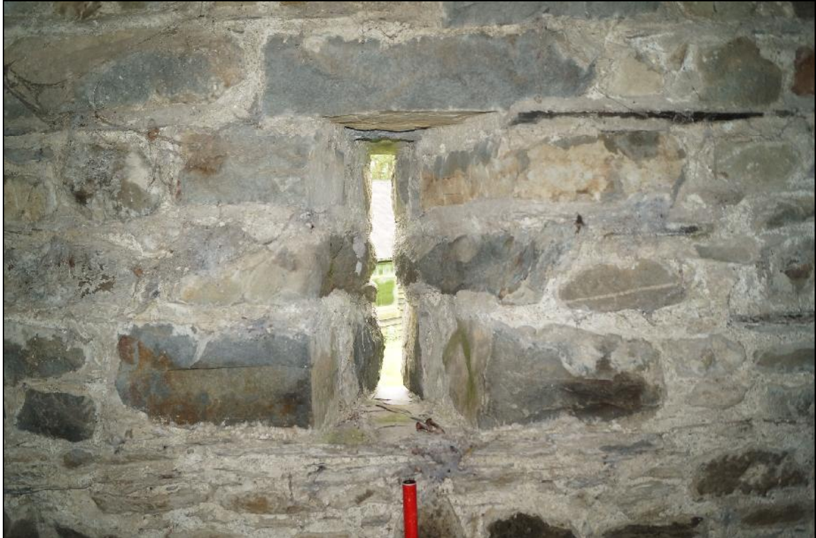
Plate 127: CYD2018_127, a closer view of the northern slit window in the western wall of the barn, looking west.
