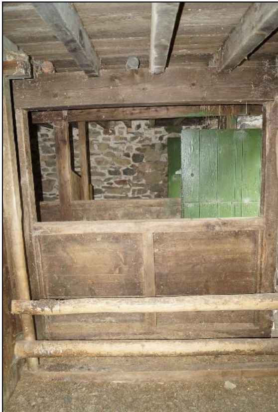
Plate 58: CYD2018_058, internal view of the cowshed, showing the eastern feeding stall at the southern end of the cowshed and looking north-northwest, with the doors into the northern stalls and the central passageway behind.
