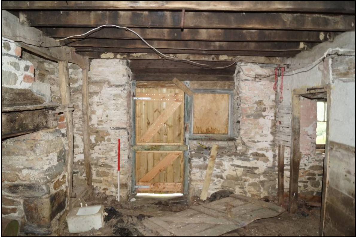
Plate 85: CYD2018_085, an interior view of the kitchen at Cwmclyd, looking west-southwest and showing the western door into the building.
